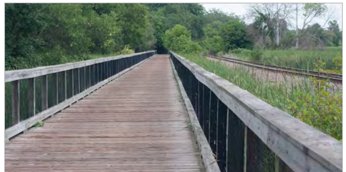
Boardwalk segment of Luce Line Regional Trail near Medicine Lake. Photo credit: SRF Consulting Group
