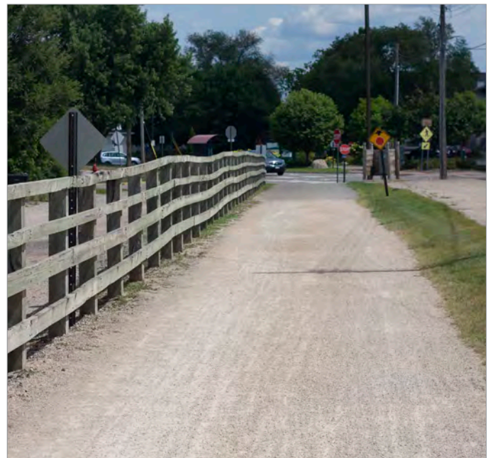
Minimum clear zone clearance is not being achieved near 9th Avenue North. Photo credit: SRF Consulting Group
