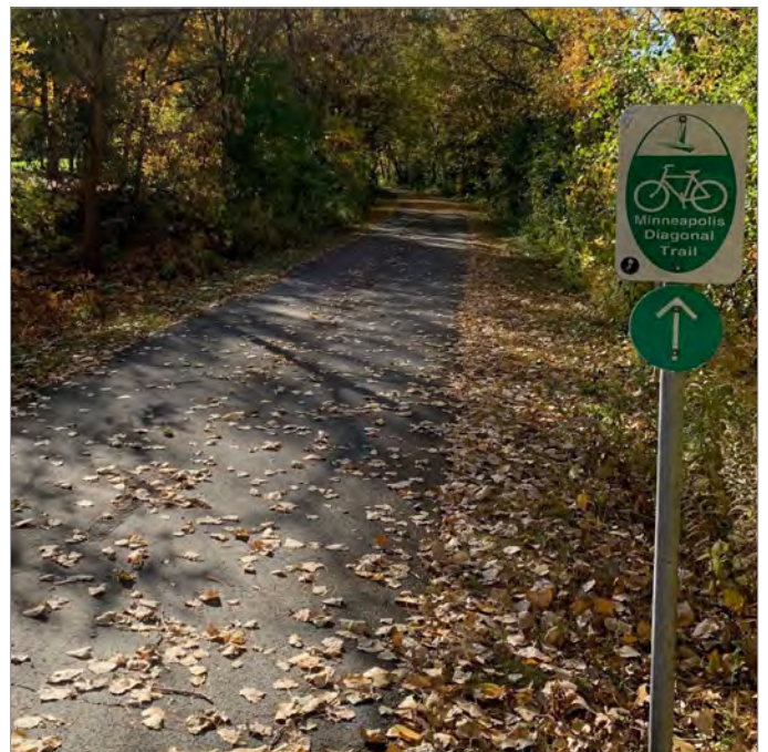
This area of the Northeast Diagonal LRT Regional Trail has segment with poor drainage. Photo credit: SRF Consulting Group
