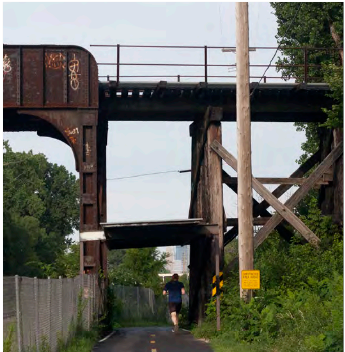
The tight railroad right-of-way creates clear zone compliance issues, as seen here under the railroad bridge overpass. Photo credit: SRF Consulting Group
