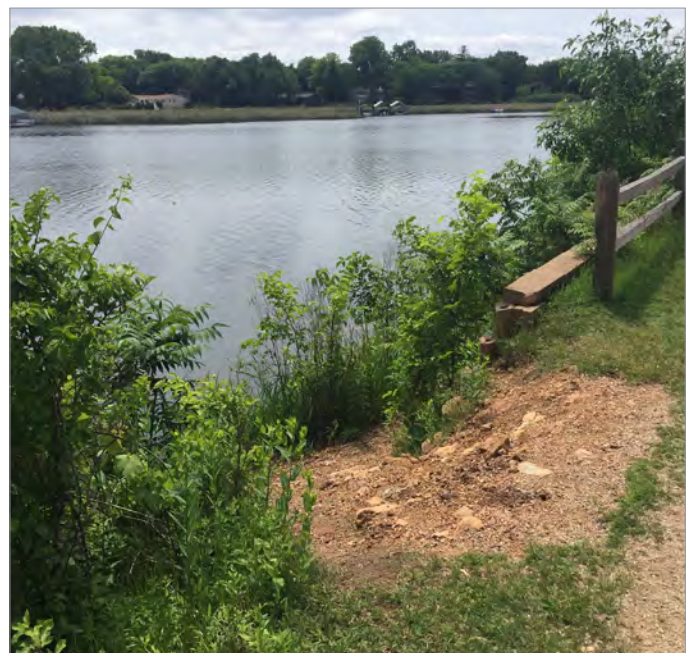
Observed erosion near the corner of the bridge. Photo credit: SRF Consulting Group
