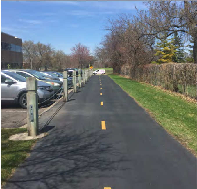
No clear zone adjacent to trail between Country Club Drive and Golden Valley Road. Photo credit: SRF Consulting Group
