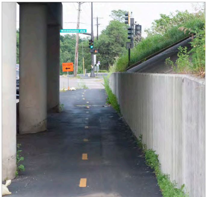
Narrow and poor pavement condition under TH 169. Photo credit: SRF Consulting Group
