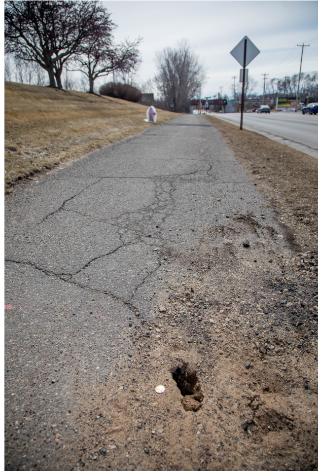
Figure 12 Cracking and pothole on Medicine Lake Regional Trail
