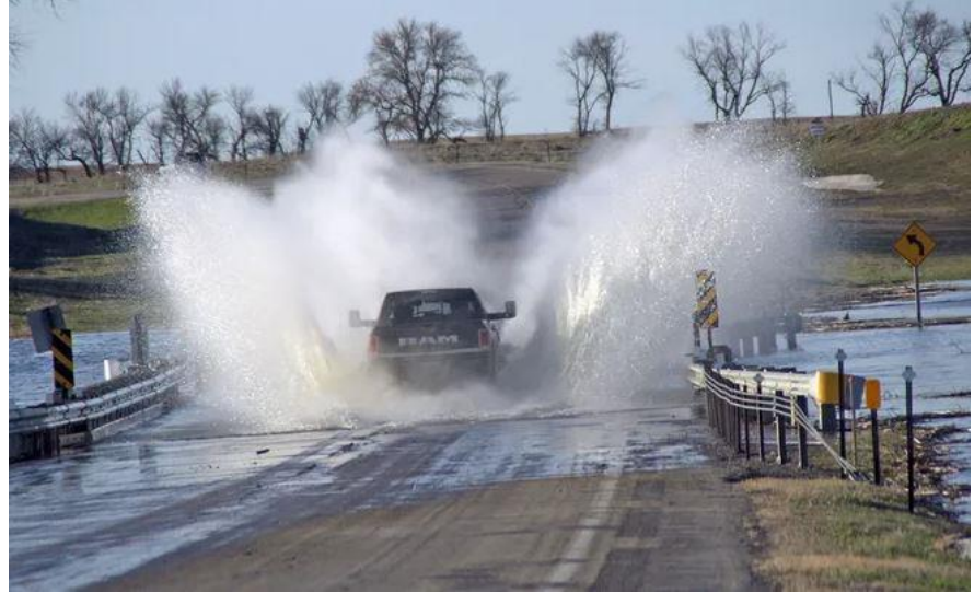
Figure 3. Lake Poinsett Outlet Bridge Deck Flooding, Spring 2019 (Watertown Public Opinion)
