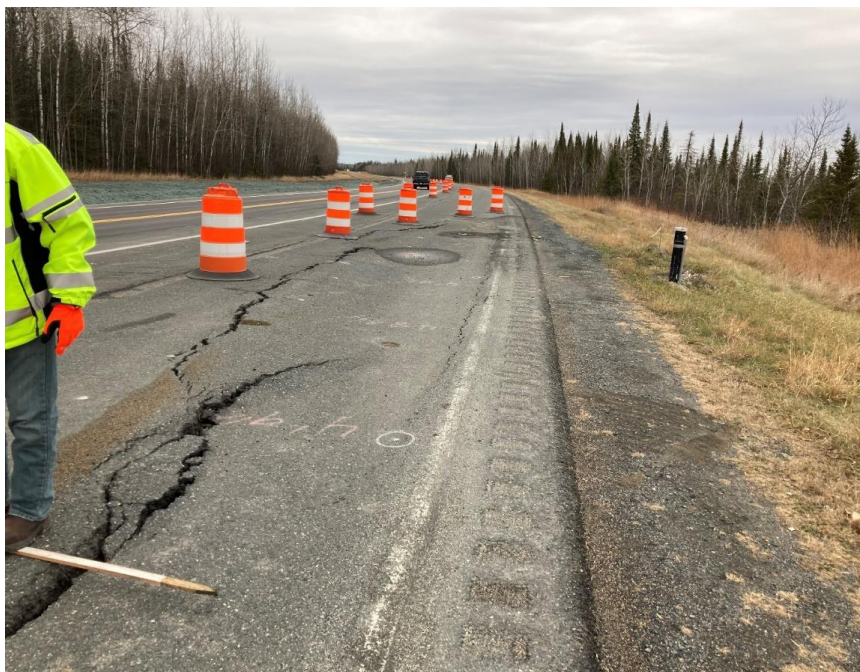
Figure 4. Slope Instability After Emergency Measures Were Taken
