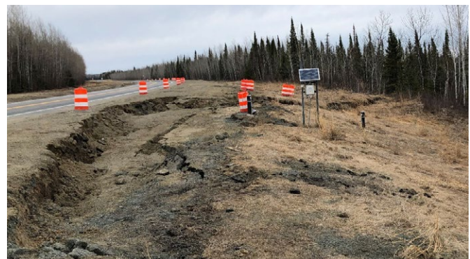
This remote monitoring system has allowed MnDOT to closely monitor the horizontal displacement of the slide area.
