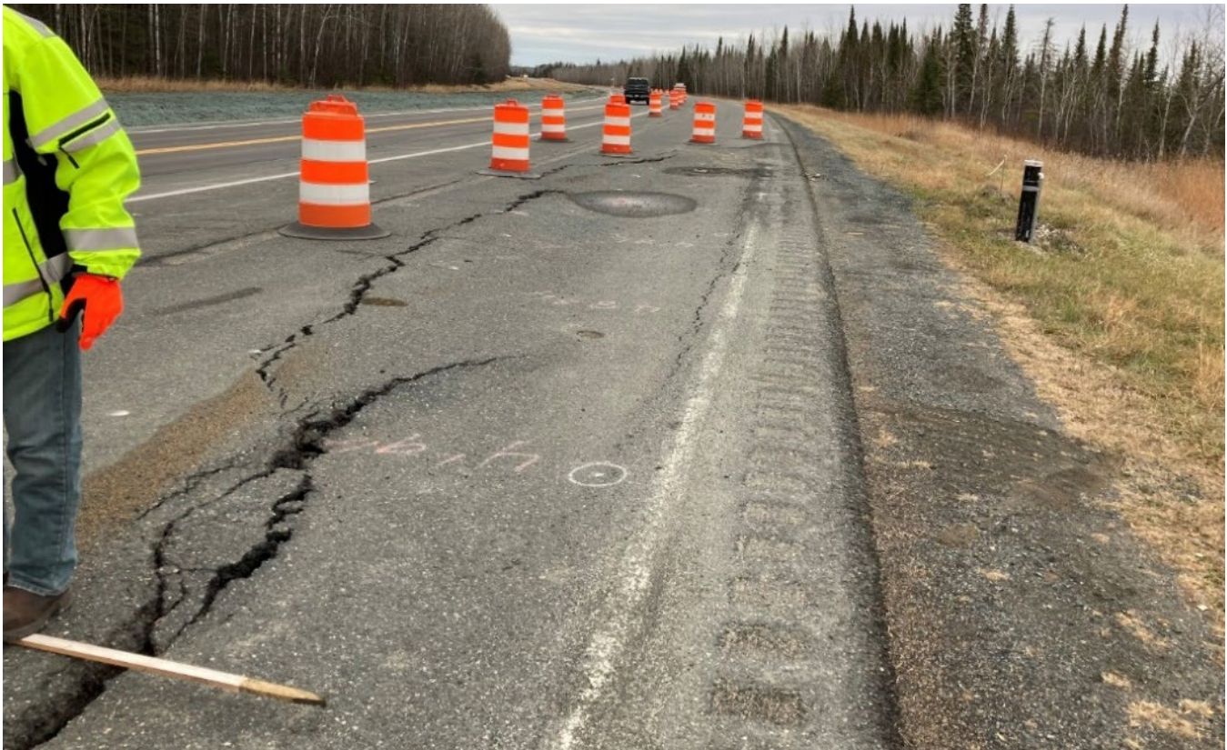
North slide area, showing the impacts to the original road from the slide. To temporarily mitigate the impacts to the roadway, MnDOT shifted Highway 11 about 20 feet west, which can be seen on the left side of this photograph.
