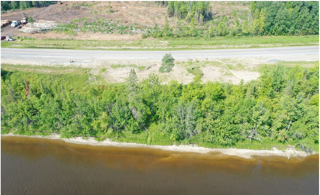
North Slide Area on in early August 2023. Despite temporary action taken by MnDOT in Fall of 2022, the slide continues to move at a concerning rate.
