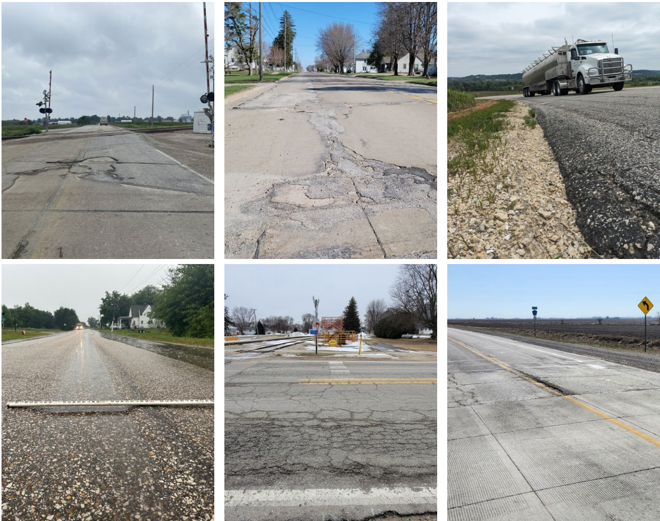
Figure 3 Current Infrastructure Conditions
