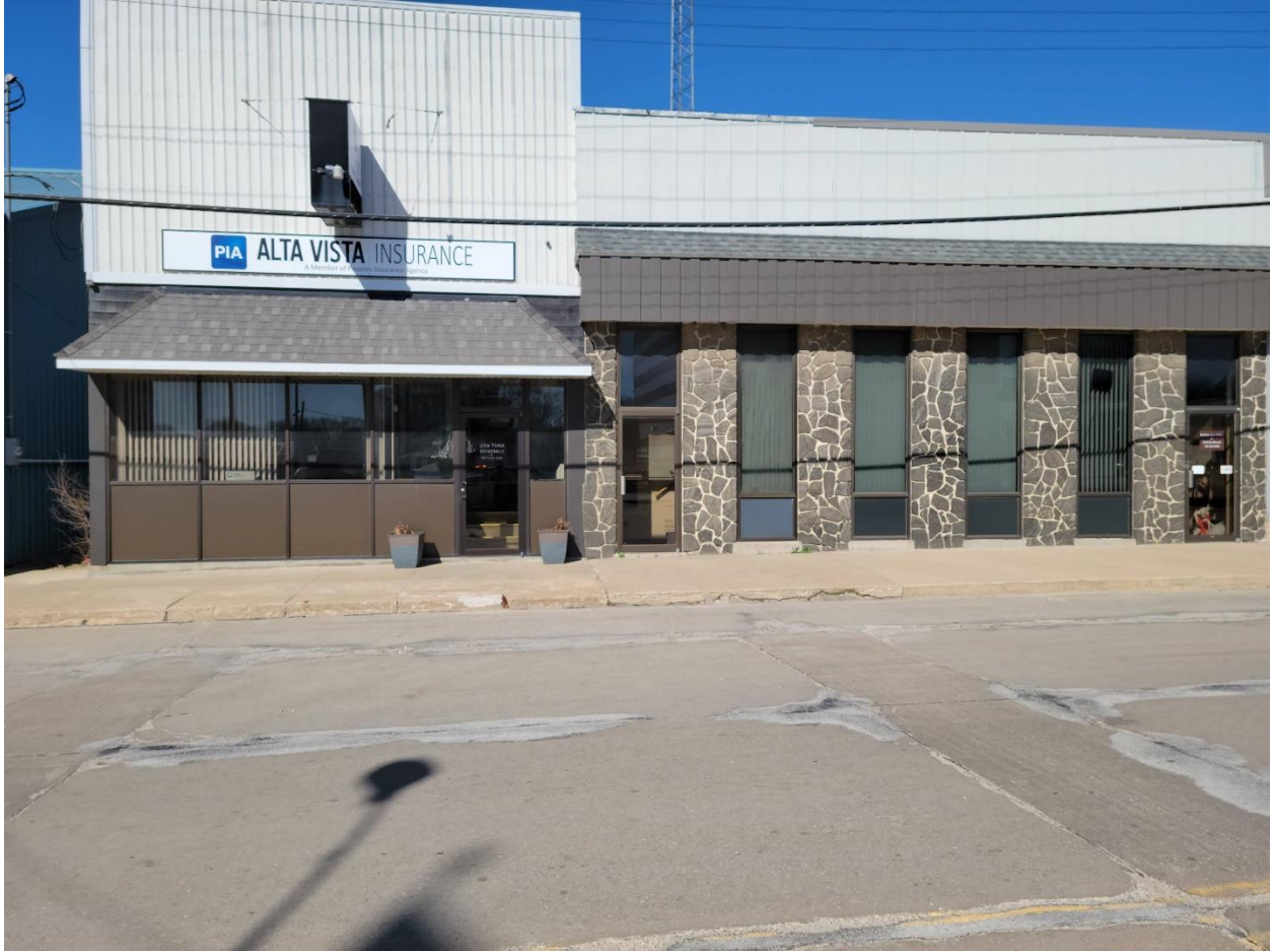
Figure 29: South White St. existing pavement deterioration next to Security State Bank/Alta Vista Insurance (Facing West)
