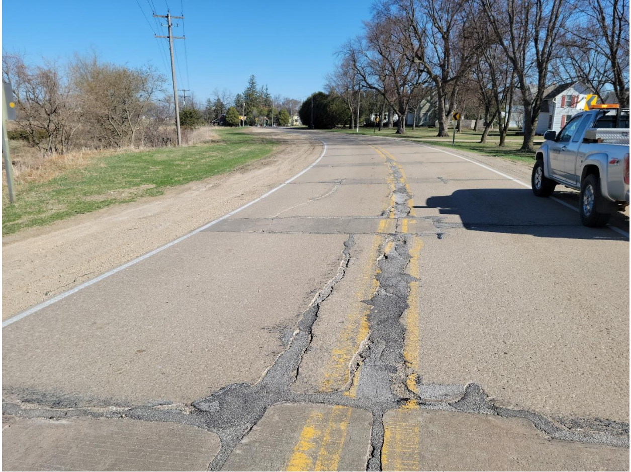
Figure 2: V18/South White St. Typical Pavement Deterioration (Facing North)
