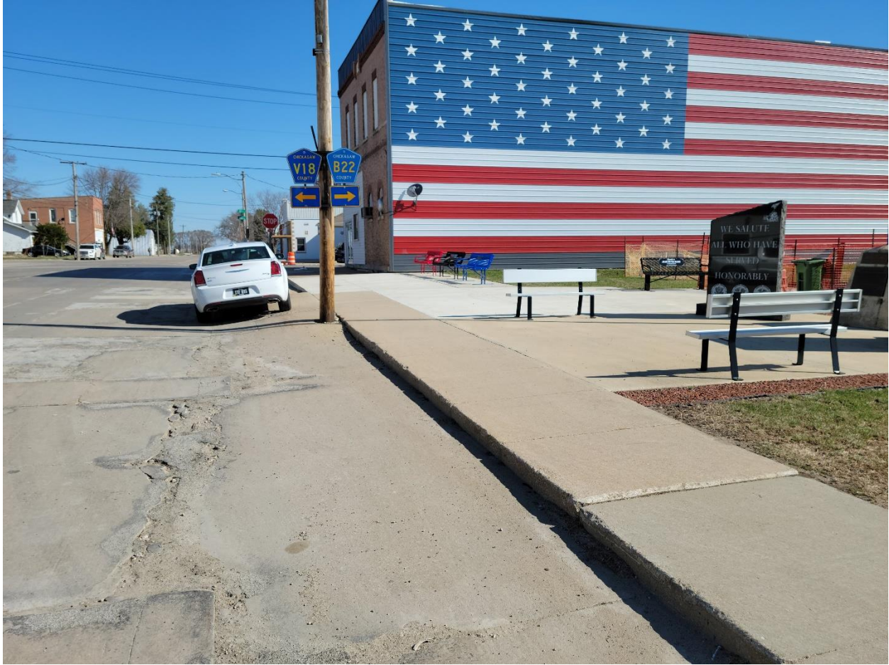
Figure 24: South White St. existing pavement deterioration/sidewalk/curb next to Linden Park/Veterans Memorial (Facing Northeast)
