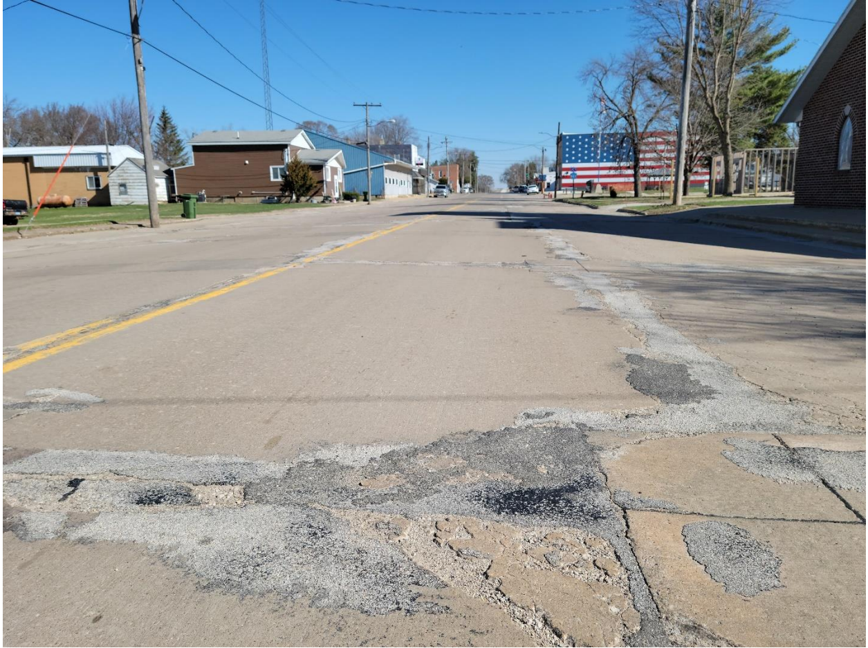
Figure 21:South White St. existing pavement deterioration (Facing North)
