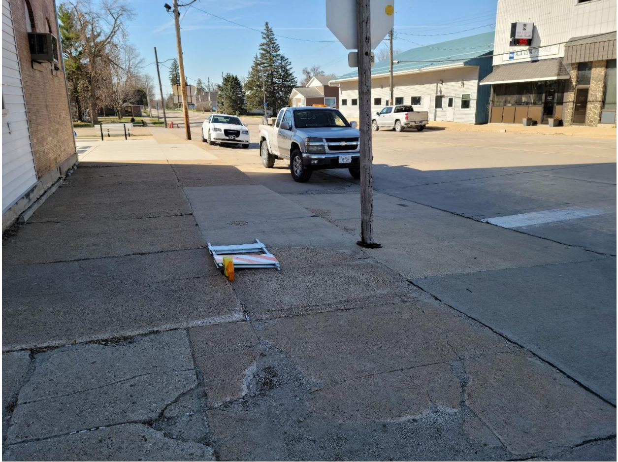
Figure 35: Existing sidewalk at Southeast corner of South White St./Weber St. Intersection next to Schuckys Bar & Grill (Facing Southwest)
