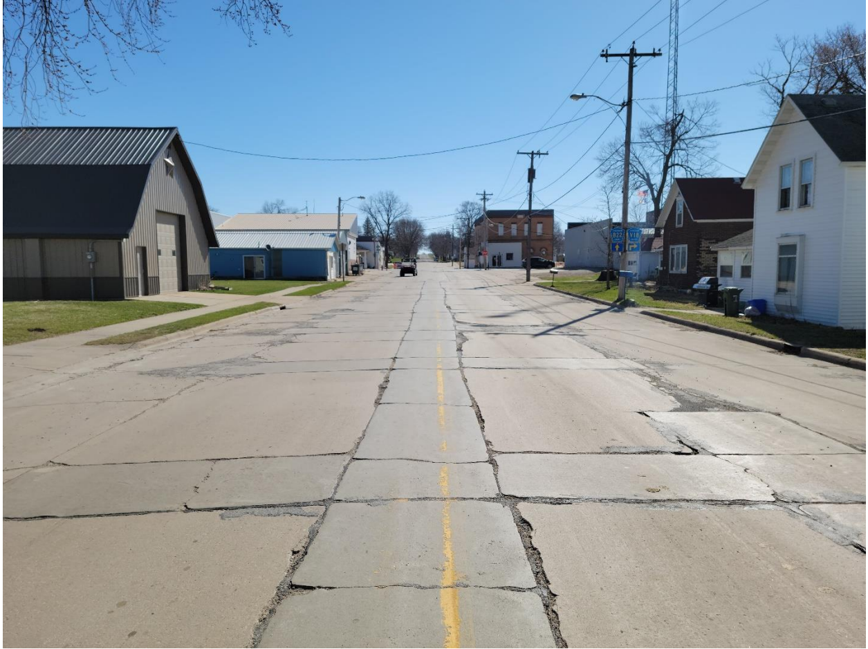
Figure 44: Weber St. existing pavement deterioration (Facing East)
