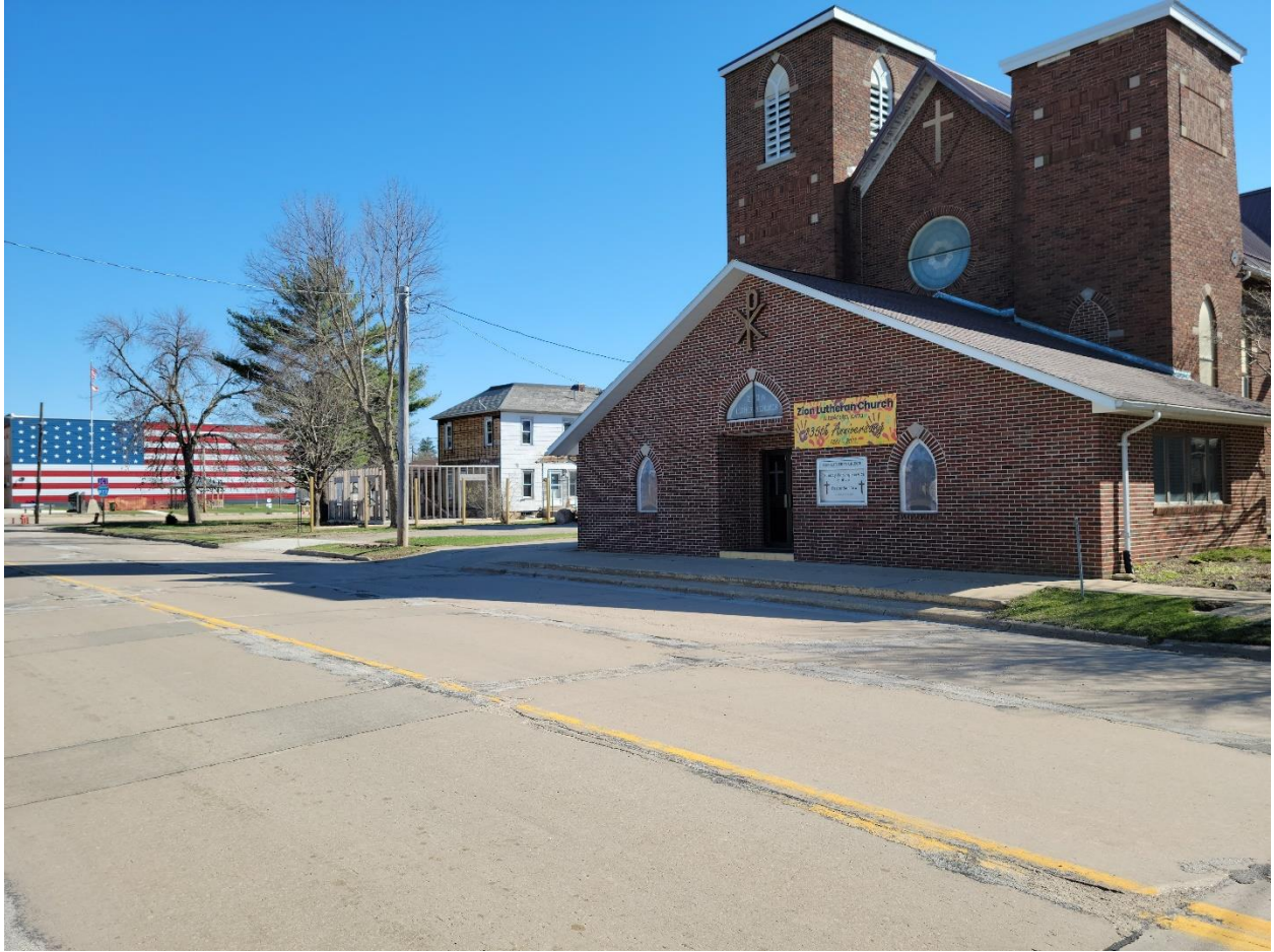
Figure 20: Existing pavement deterioration next to Zion Lutheran Church (Facing Northeast)
