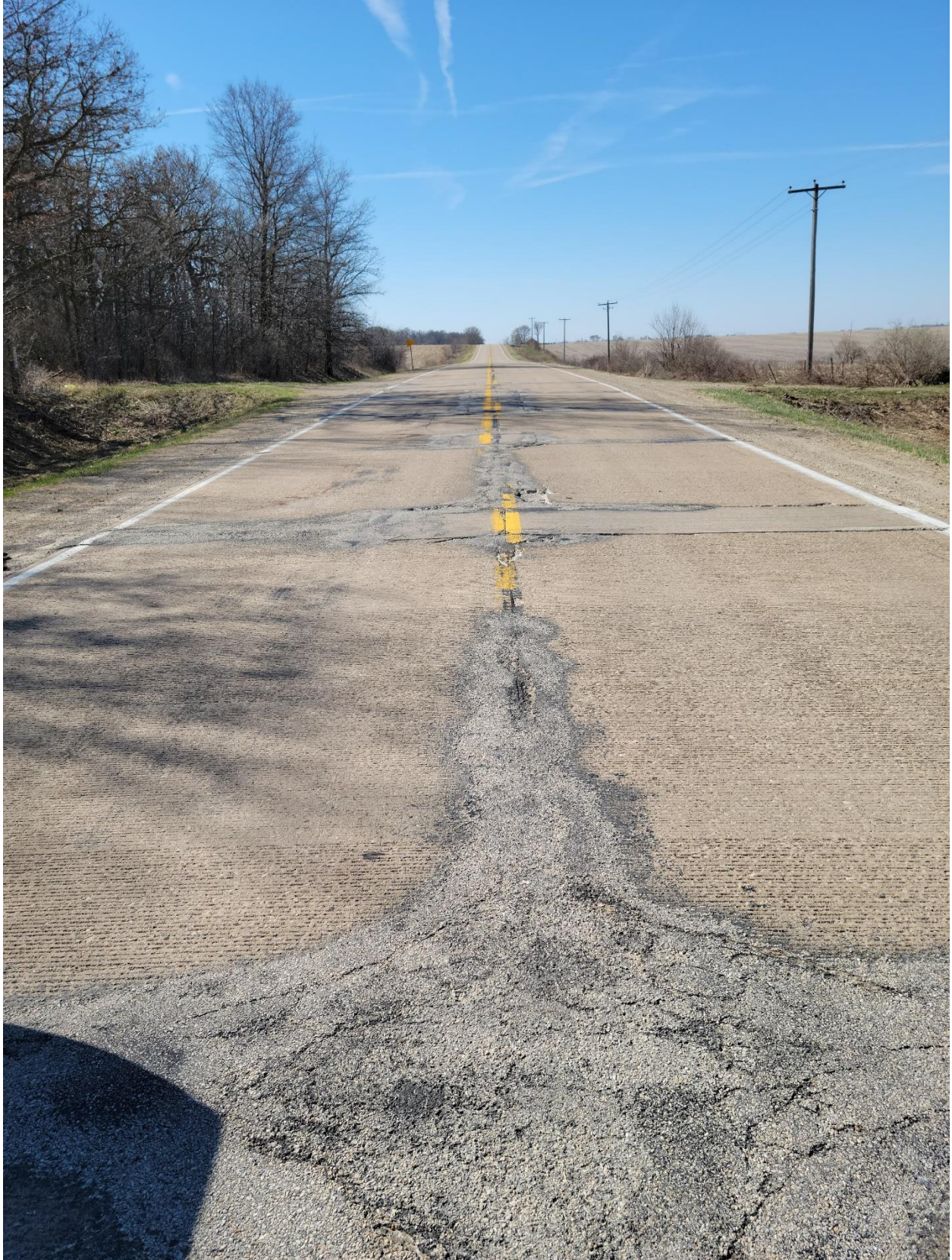
Figure 52:v18/Fayette Ave. existing pavement deterioration (Facing South)
