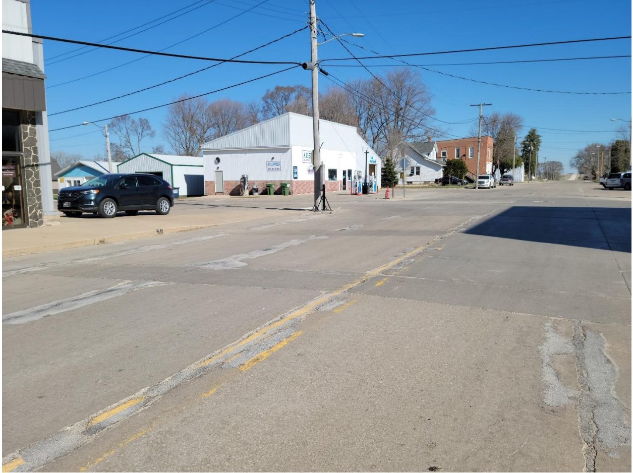
Figure 28:South White St./Weber St. intersection existing pavement deterioration next to A.V. Express Gas Station (Facing North)
