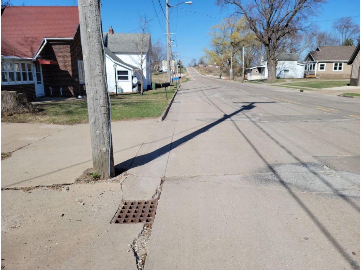
Figure 42: Weber St. existing pavement deterioration/intake (Facing West)
