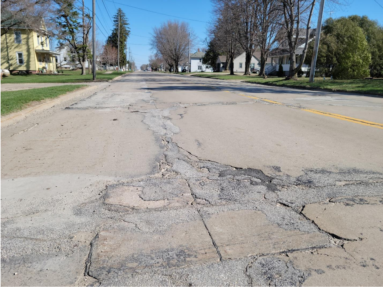
Figure 6: South White St. typical pavement deterioration (Facing North)
