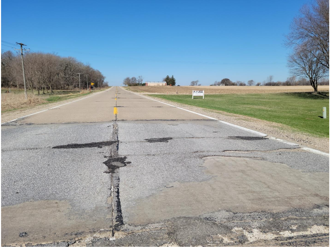
Figure 48: V18/110th St. existing pavement deterioration next to Dr. Z's Auto Clinic (Facing West)
