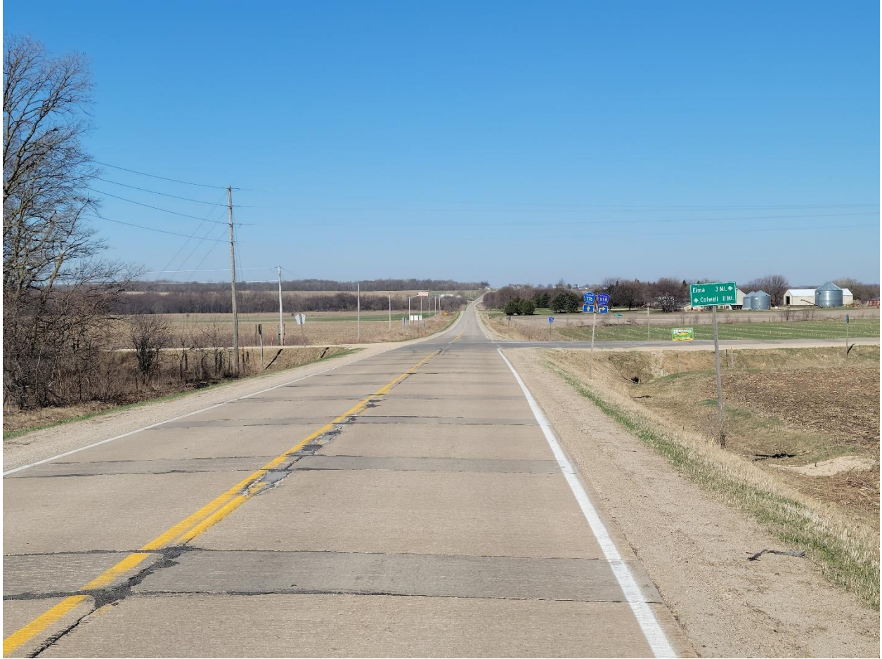
Figure 49:V18/110th St. existing pavement deterioration approaching intersection of Fayette Ave./110th St. (Facing West)
