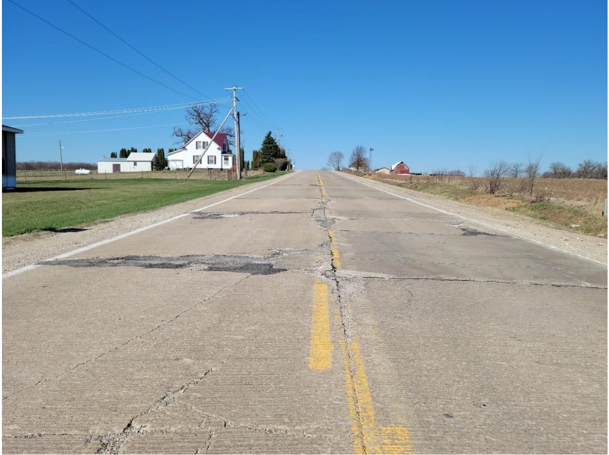
Figure 45: V18/110th St. existing pavement deterioration (Facing West)
