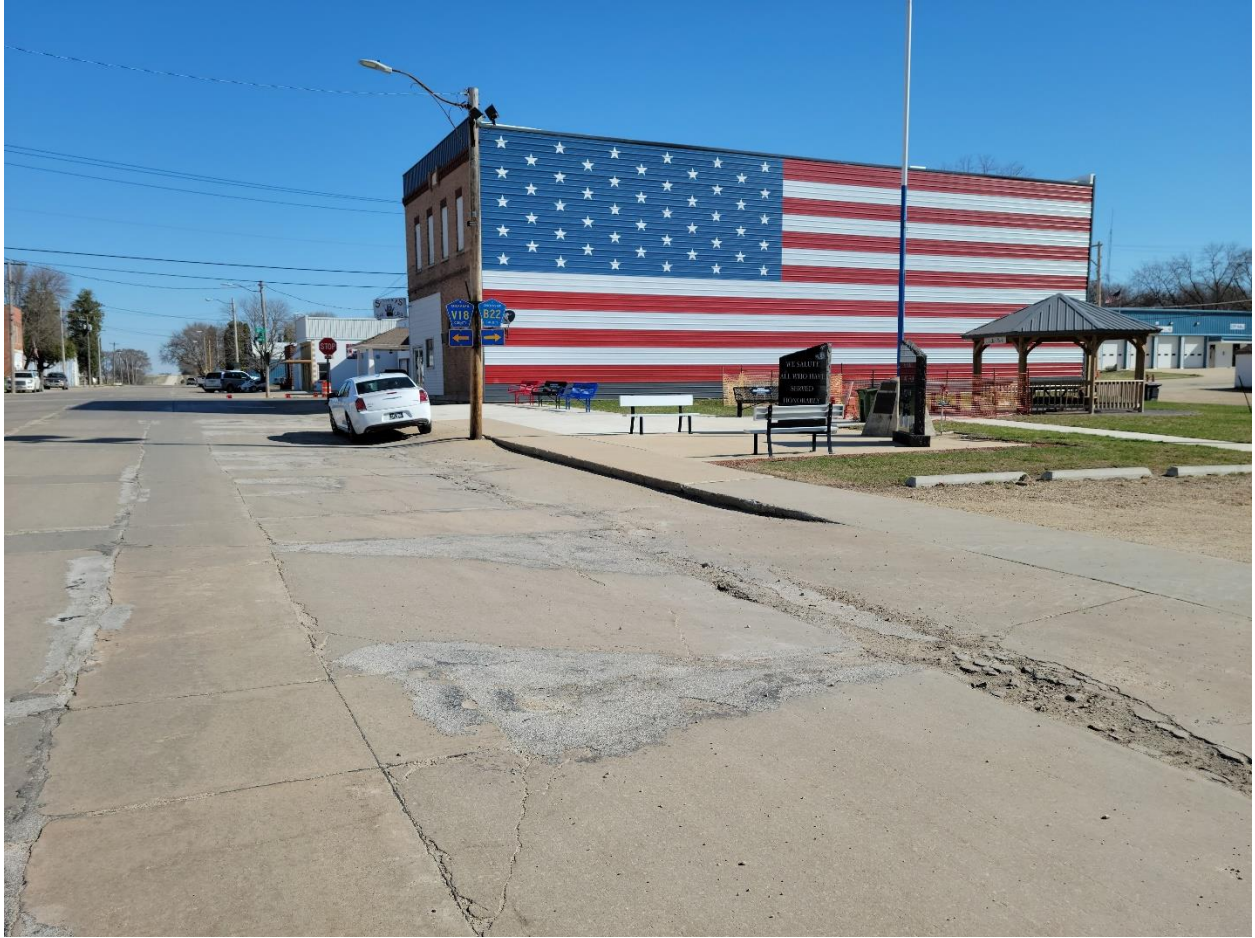
Figure 23:South White St. existing pavement deterioration next to Linden Park/Veterans Memorial (Facing Northeast)
