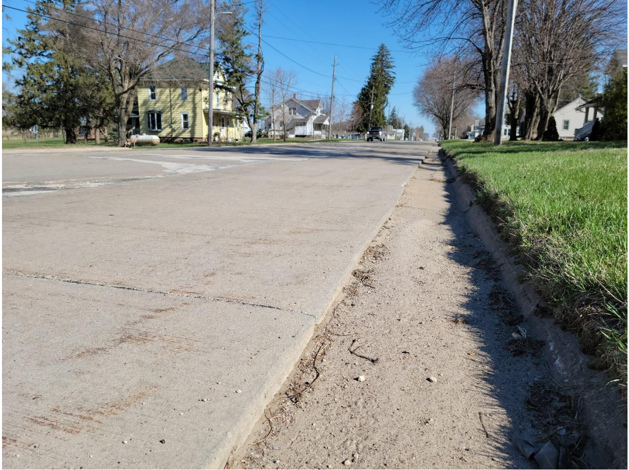
Figure 5: South White St. typical Curb/Gutter Settlement (Facing North)
