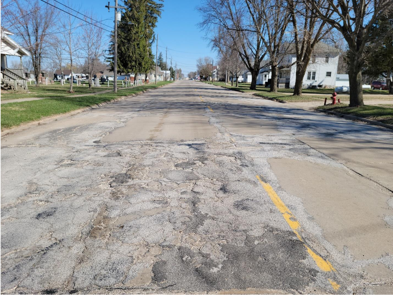
Figure 9:South White St. typical pavement deterioration (Facing North)
