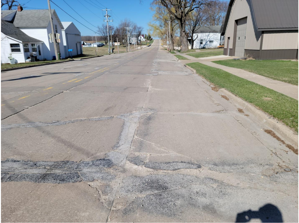
Figure 40: Weber St. existing pavement deterioration (Facing West)
