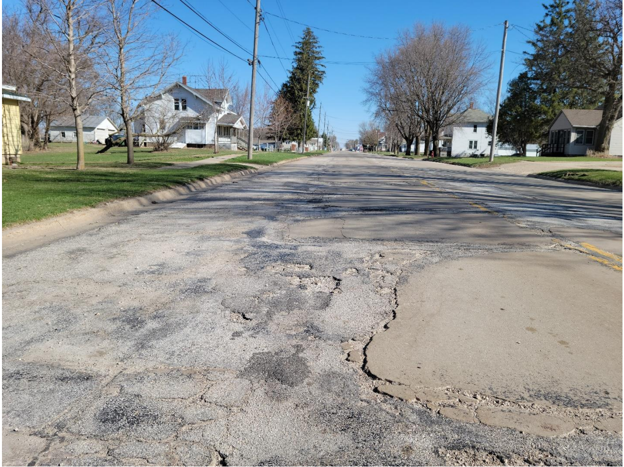
Figure 8: South White St. typical pavement deterioration (Facing North)
