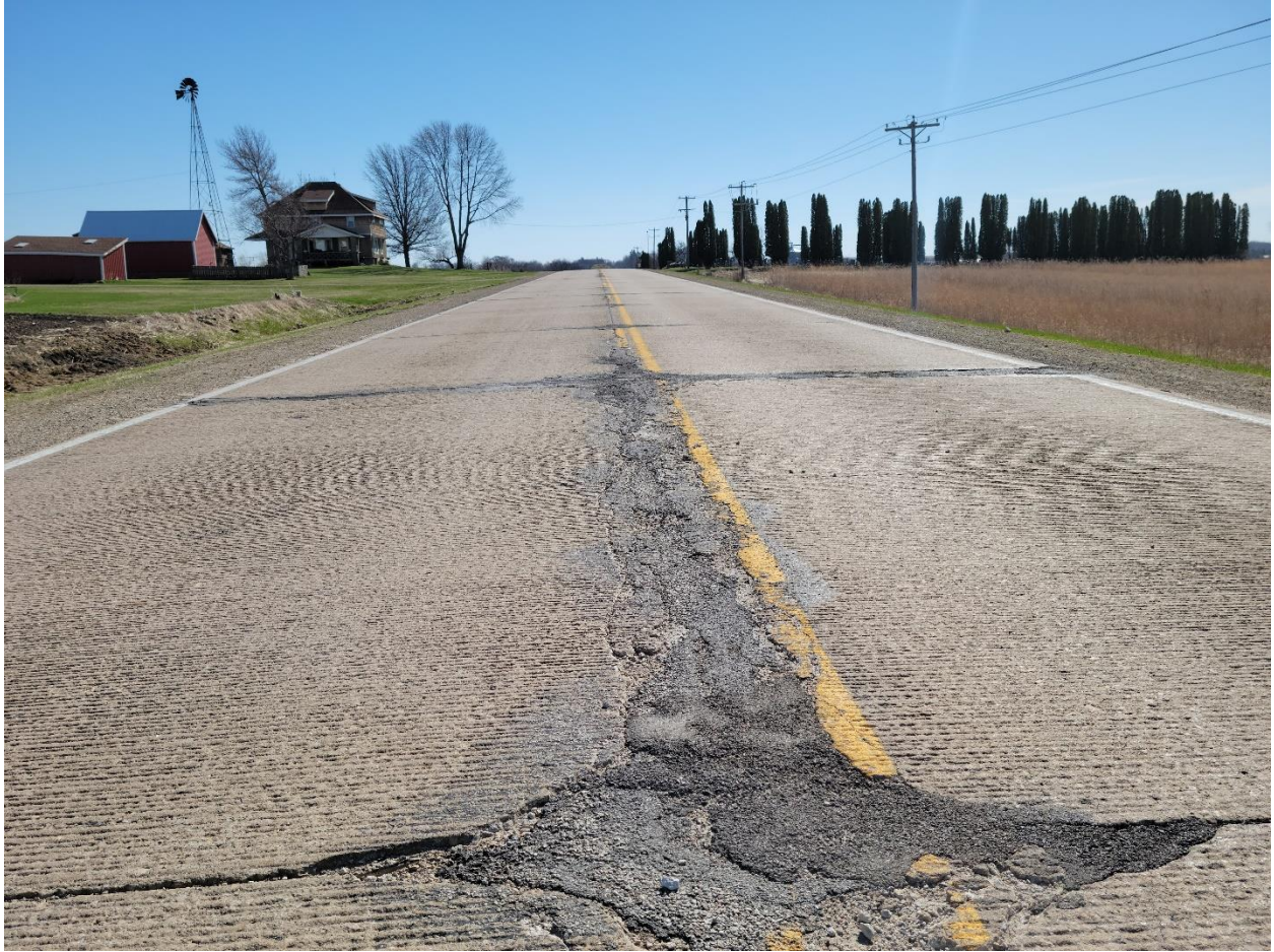
Figure 47: V18/110th St. existing pavement deterioration (Facing East)
