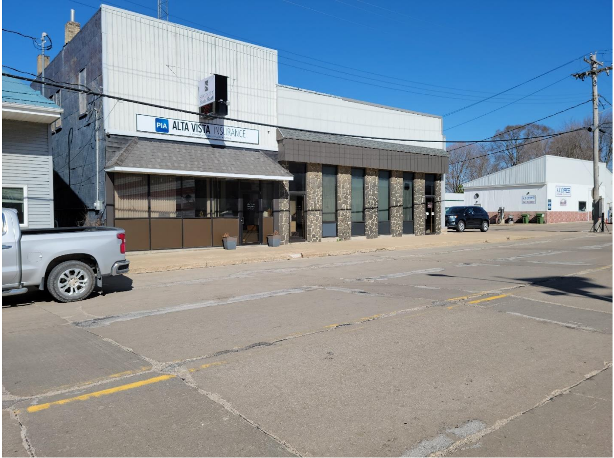
Figure 26: South White St. existing pavement deterioration next to Security State Bank/Alta Vista Insurance (Facing Northwest)
