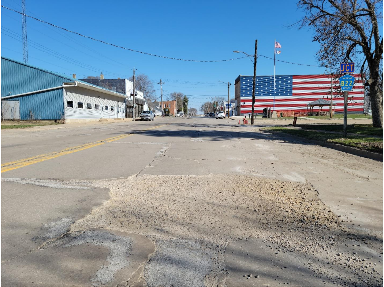
Figure 22: South White St. existing pavement deterioration (Facing North)
