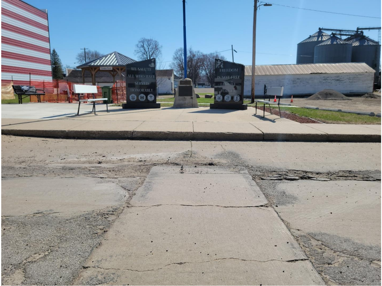
Figure 25: South White St. existing pavement deterioration/sidewalk/curb next to Linden Park/Veterans Memorial (Facing East)
