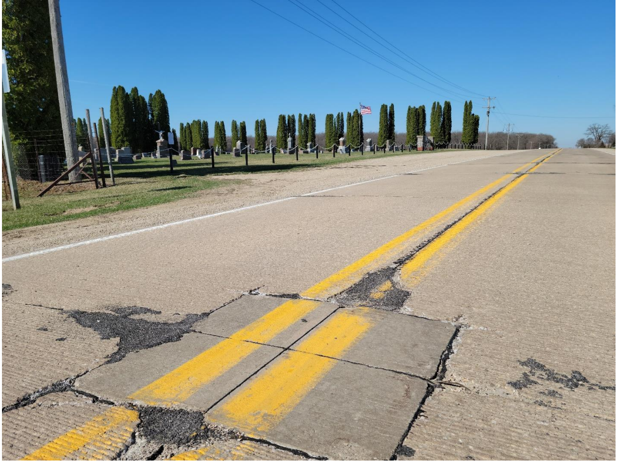
Figure 46: V18/110th St. existing pavement deterioration next to Alta Vista Cemetery (Facing Southwest)
