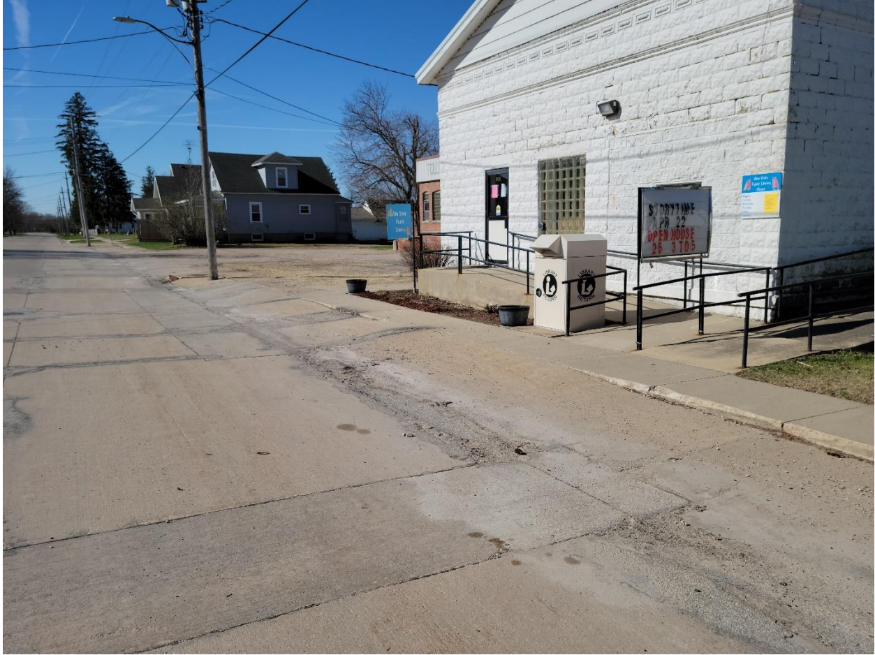
Figure 19:South White St. existing pavement deterioration/sidewalk next to Public Library (Facing Southwest)
