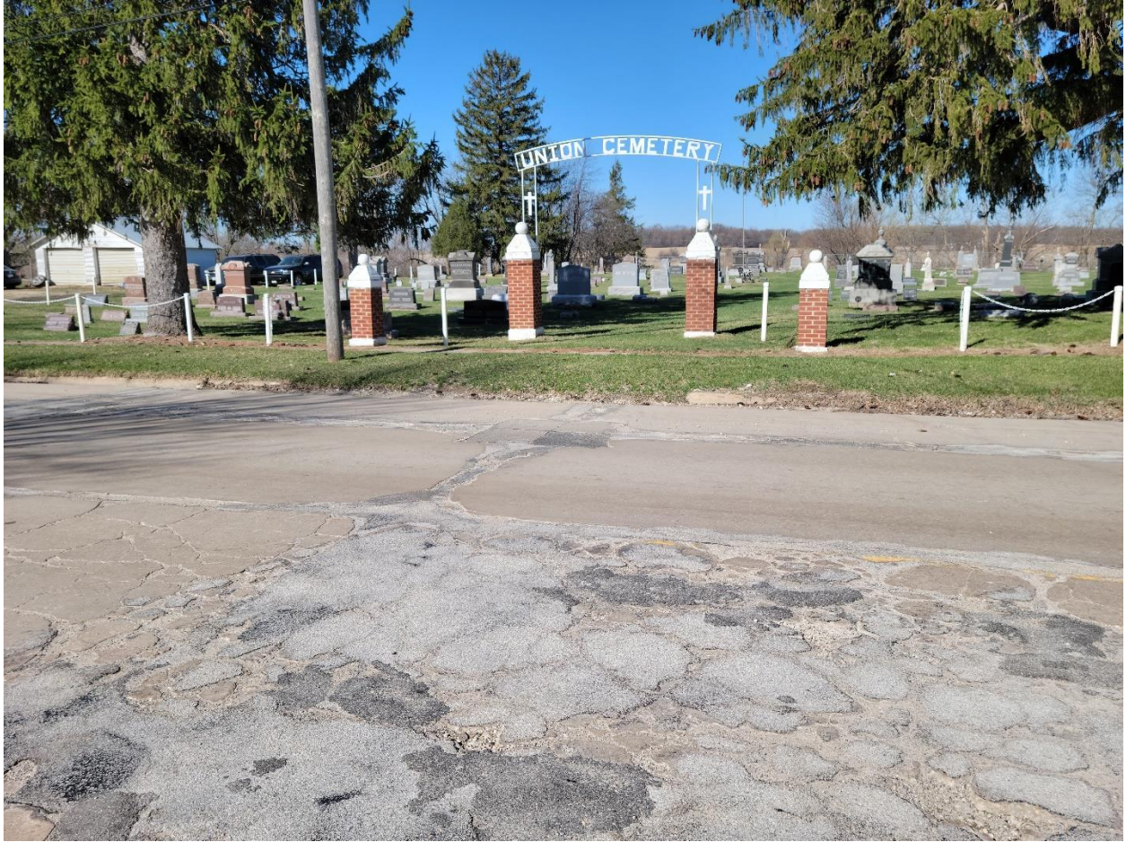
Figure 11: South White St. existing pavement deterioration at Union Cemetery entrance (Facing West)
