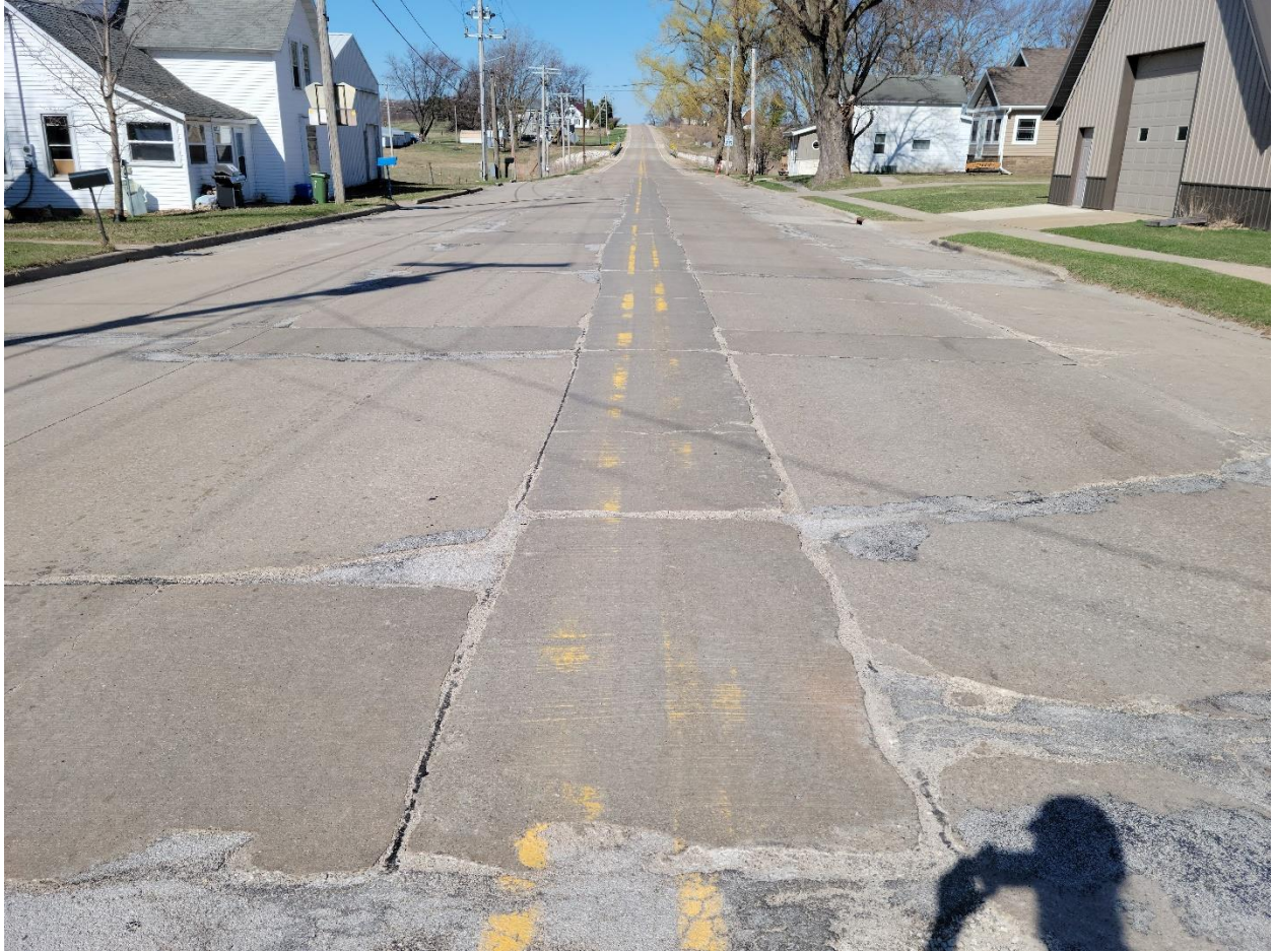
Figure 41: Weber St. existing pavement deterioration (Facing West)
