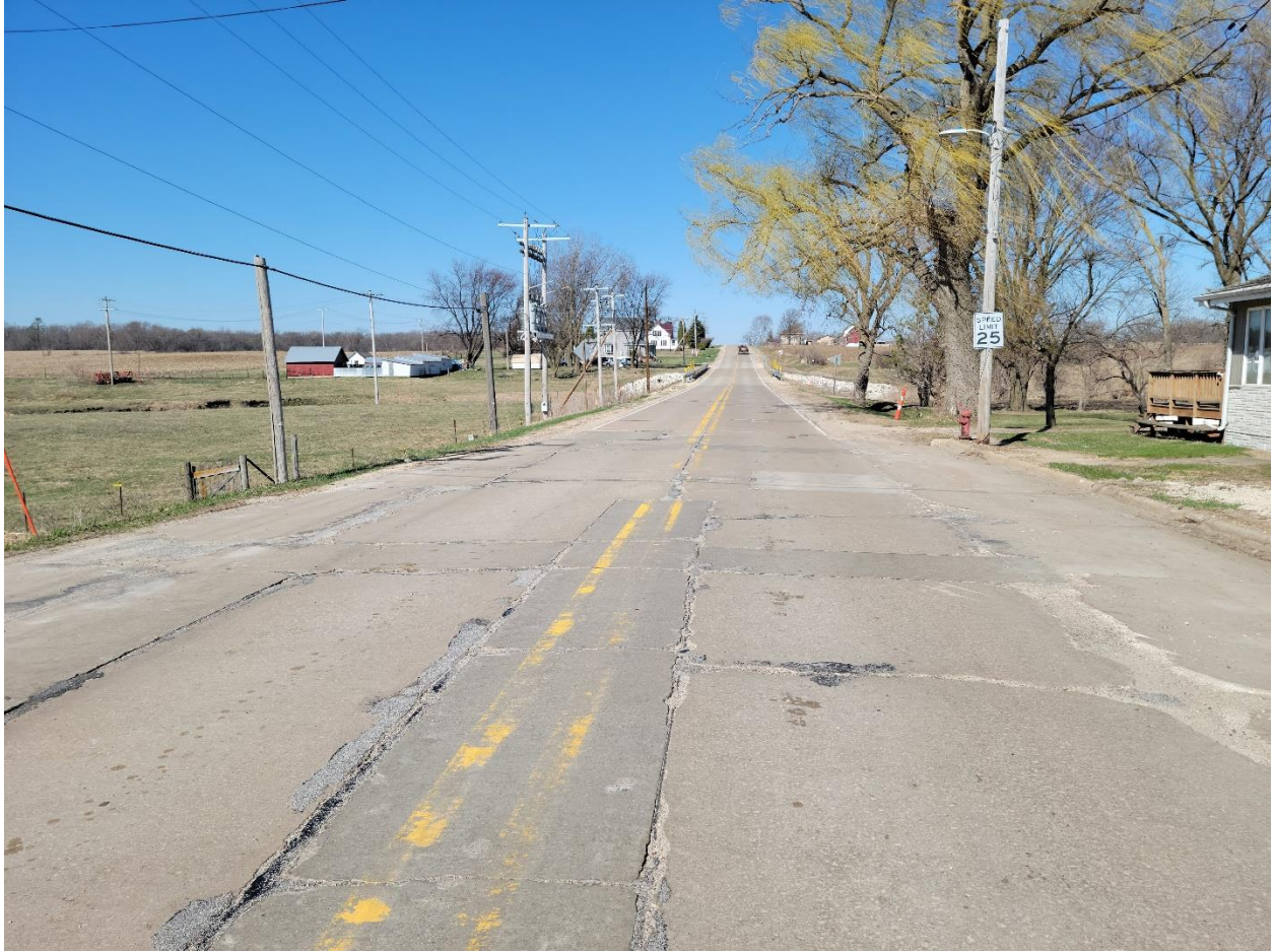
Figure 43: Weber St. existing pavement deterioration (Facing West)
