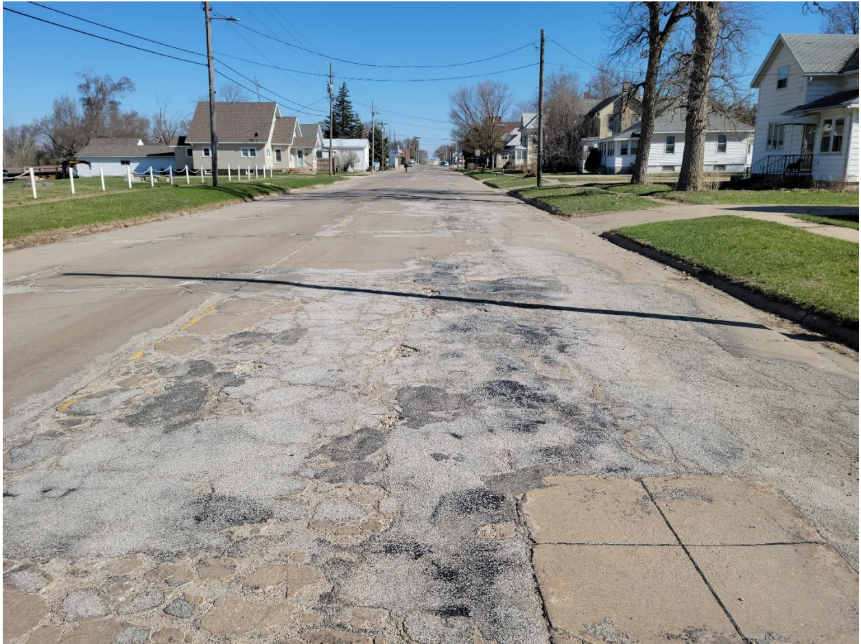
Figure 13: South White St. typical pavement deterioration (Facing North)
