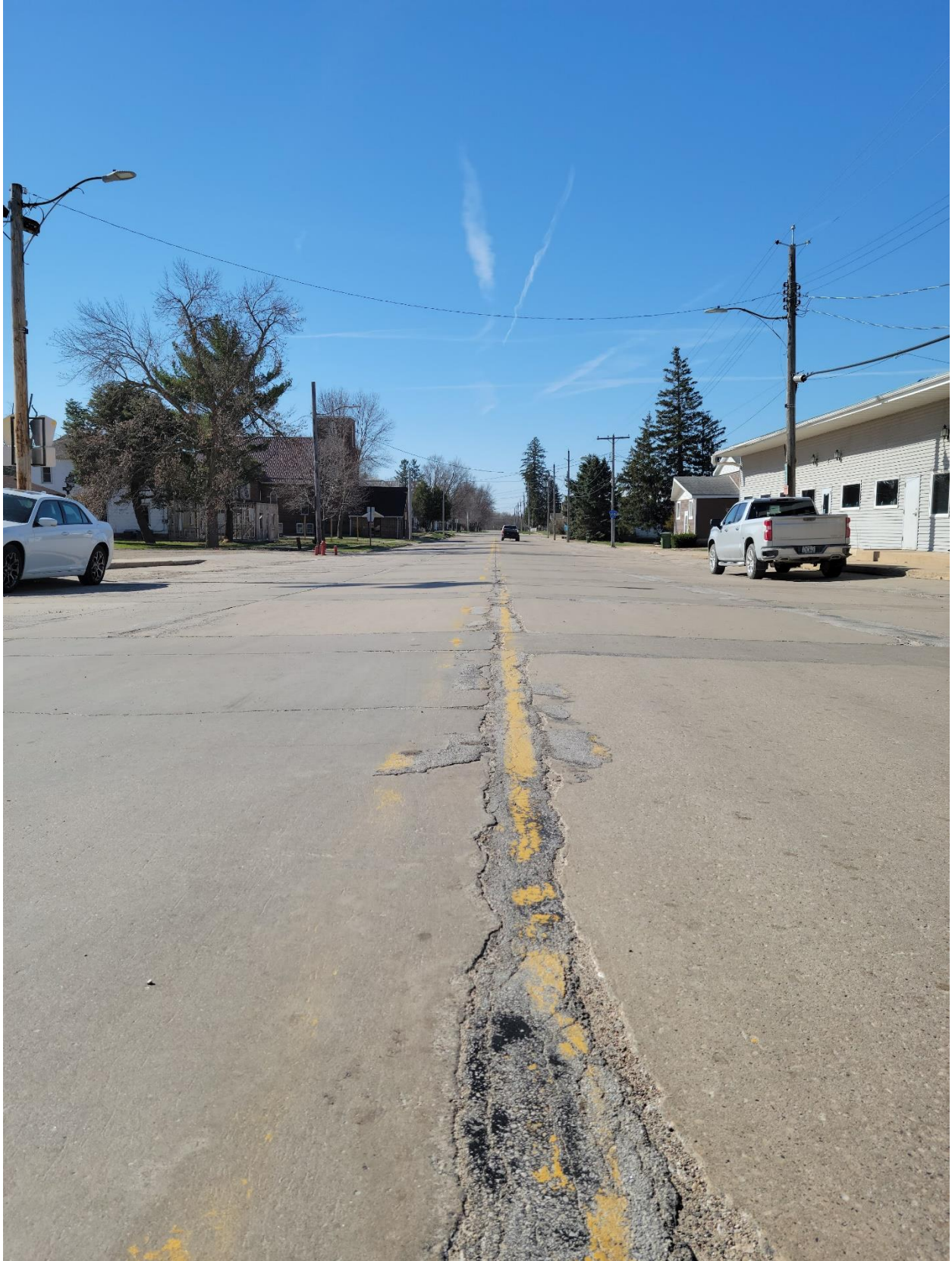
Figure 39:South White St. existing pavement deterioration (Facing South)
