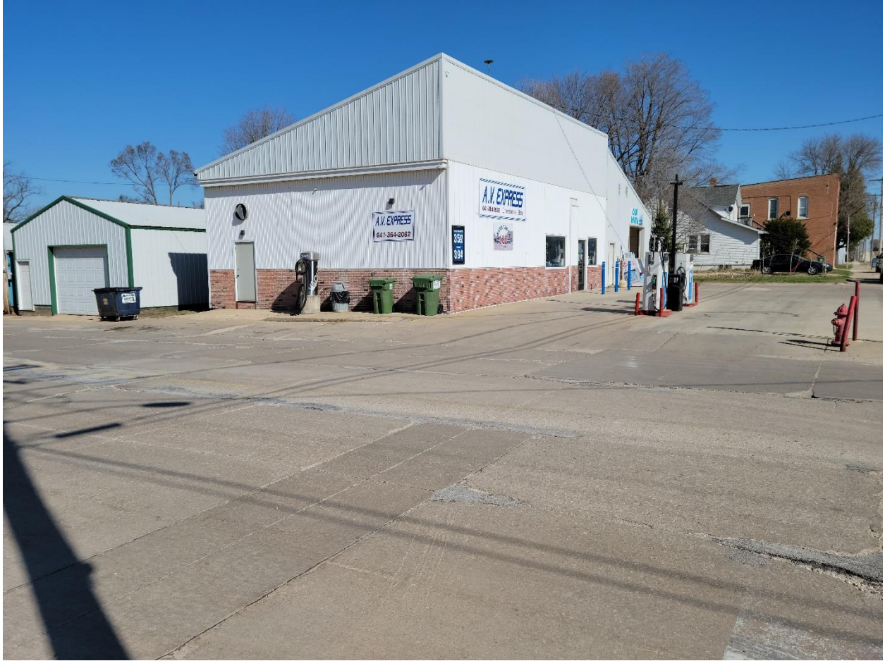
Figure 34: Weber St. existing pavement deterioration next to A.V. Express Gas Station (Facing Northwest)
