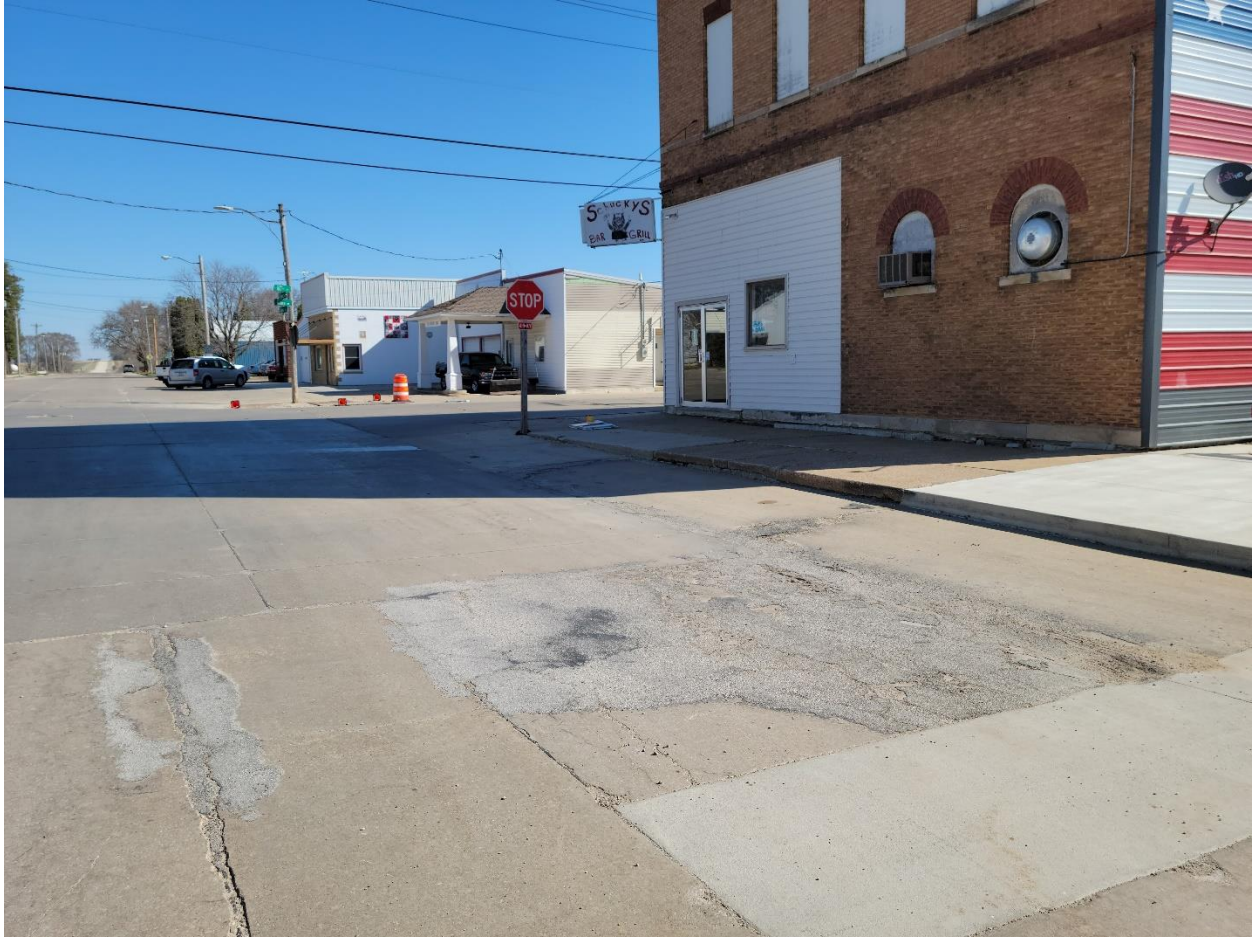
Figure 27: South White St. existing pavement deterioration next to Schuckys Bar & Grill (Facing Northeast)
