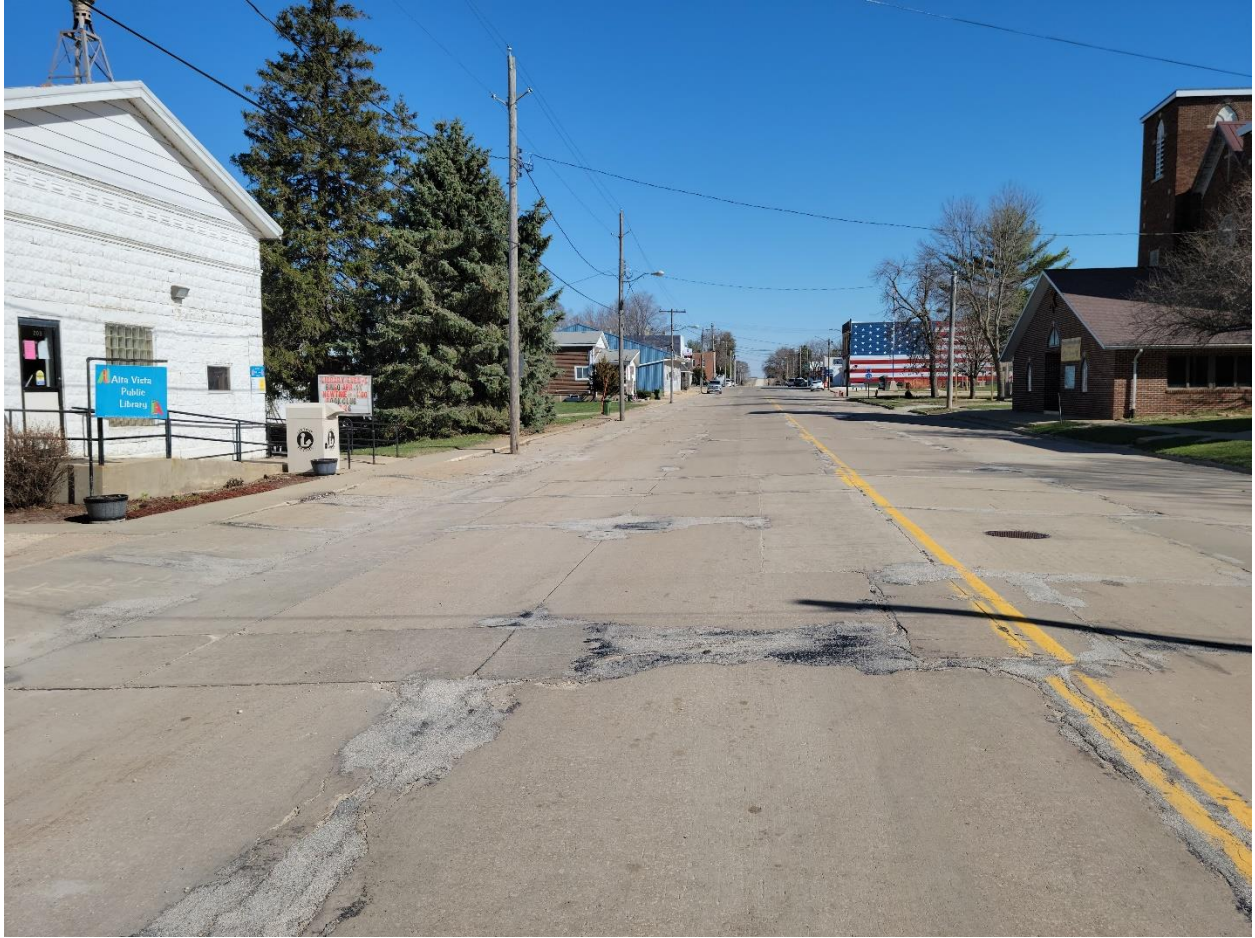
Figure 16: South White St. existing pavement deterioration next to Public Library (Facing North)
