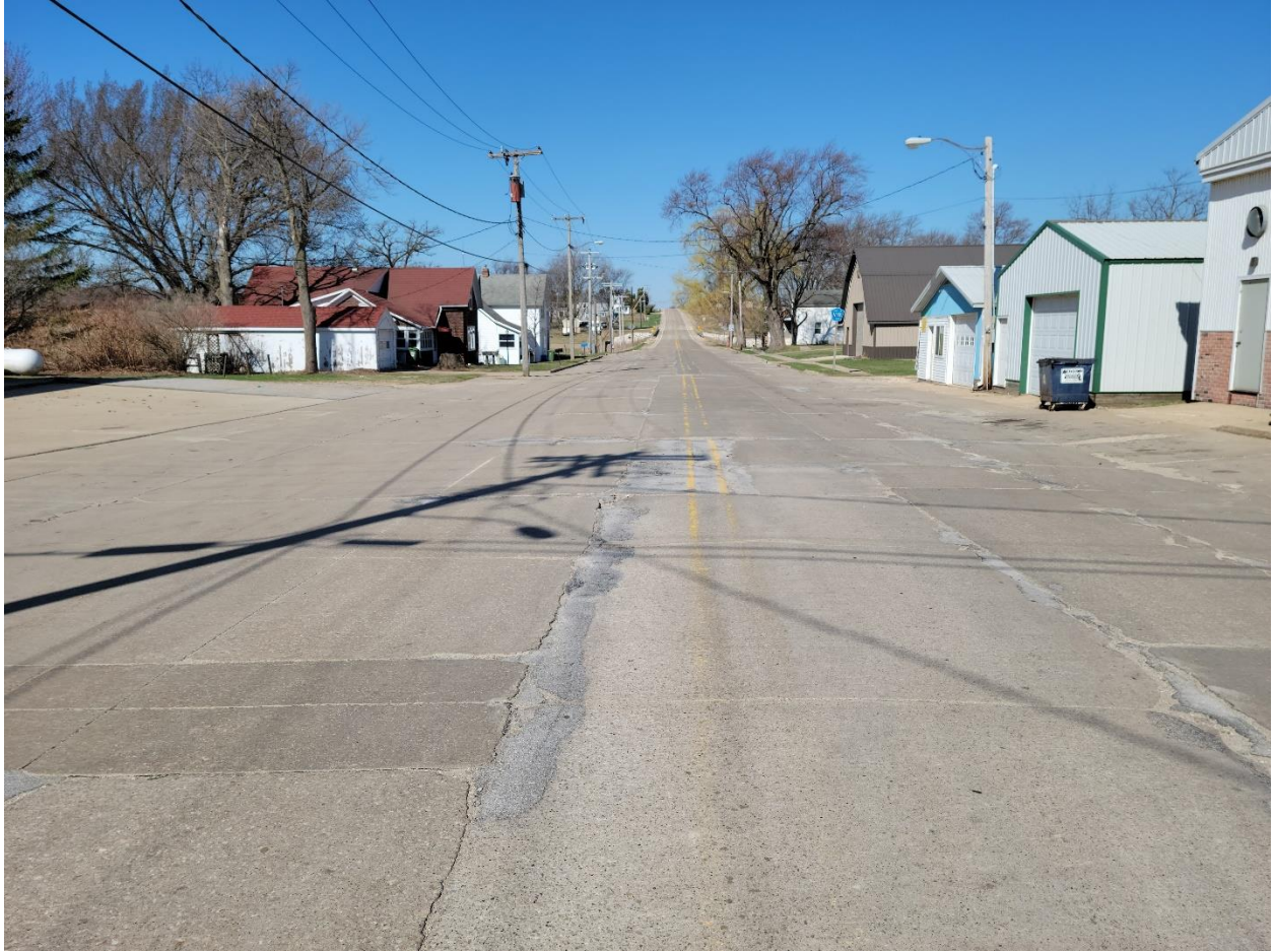
Figure 38: Weber St. existing pavement deterioration (Facing West)
