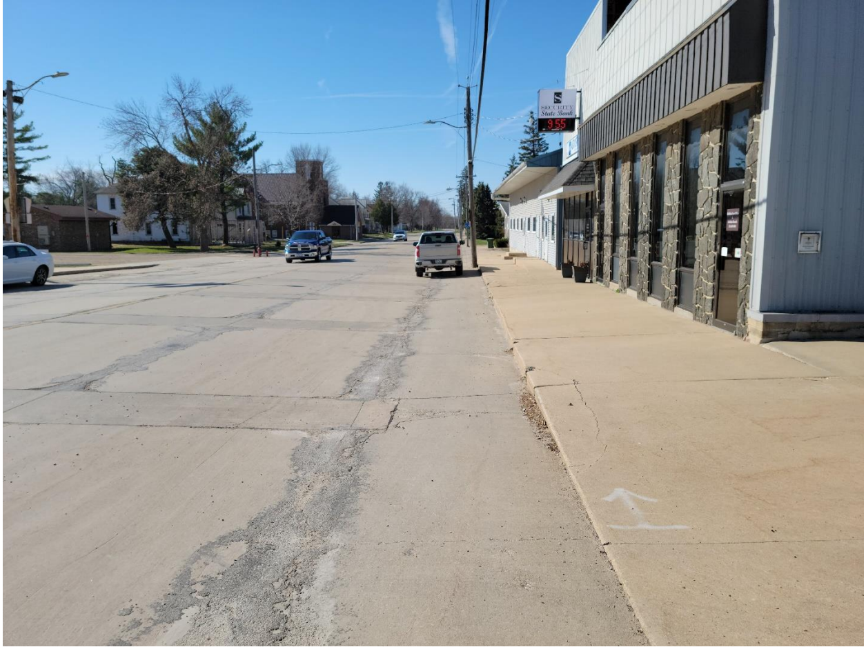
Figure 33:South White St. existing pavement deterioration/West sidewalk/curb (Facing South)
