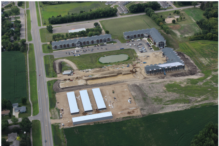
This image illustrates the Unique Opportunities development on CSAH 5 north of the project area. The Kelly Morrell storage units property is also illustrated on the south of the Unique Opportunities development.
