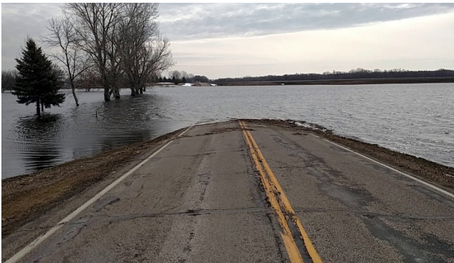
Figure 6 Flooding of the County Road 6 Bridge
