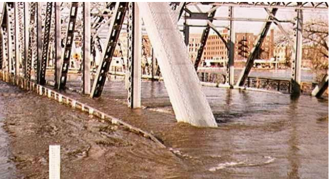
Figure 4 Flooding of 1997 - Sorlie Memorial Bridge
