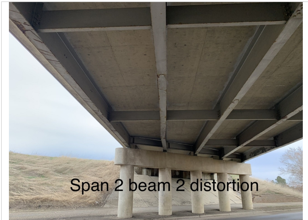
Span2 beam 2 distortion
