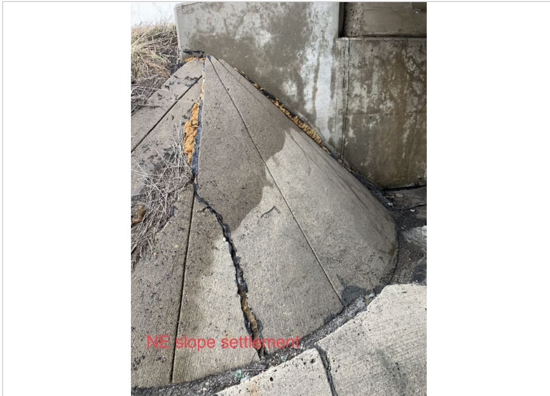
NE corner slope protection settlement
