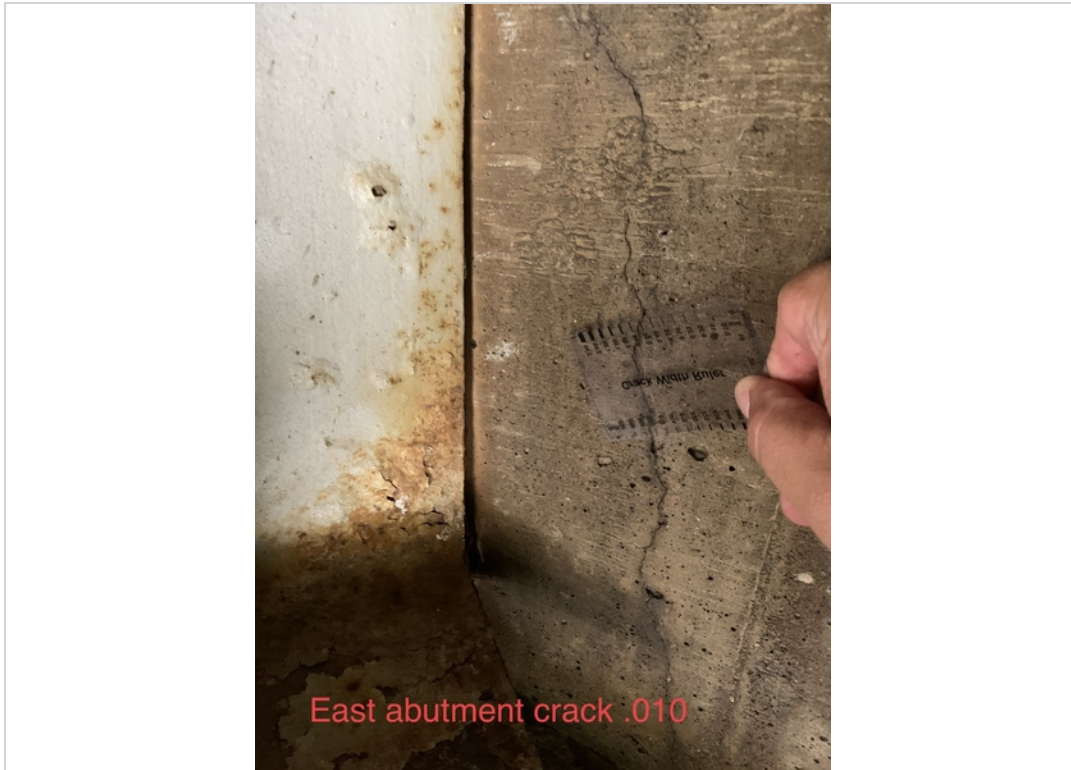
East abutment backwall crack .010
