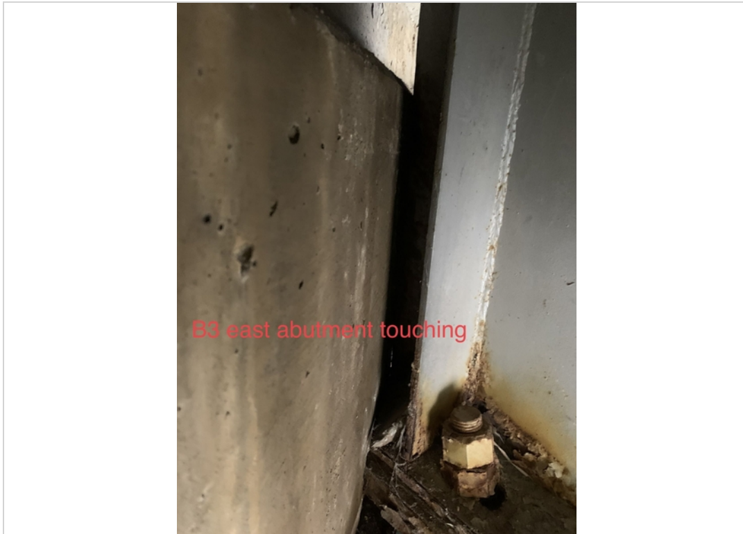
East abutment beam 3 touching
