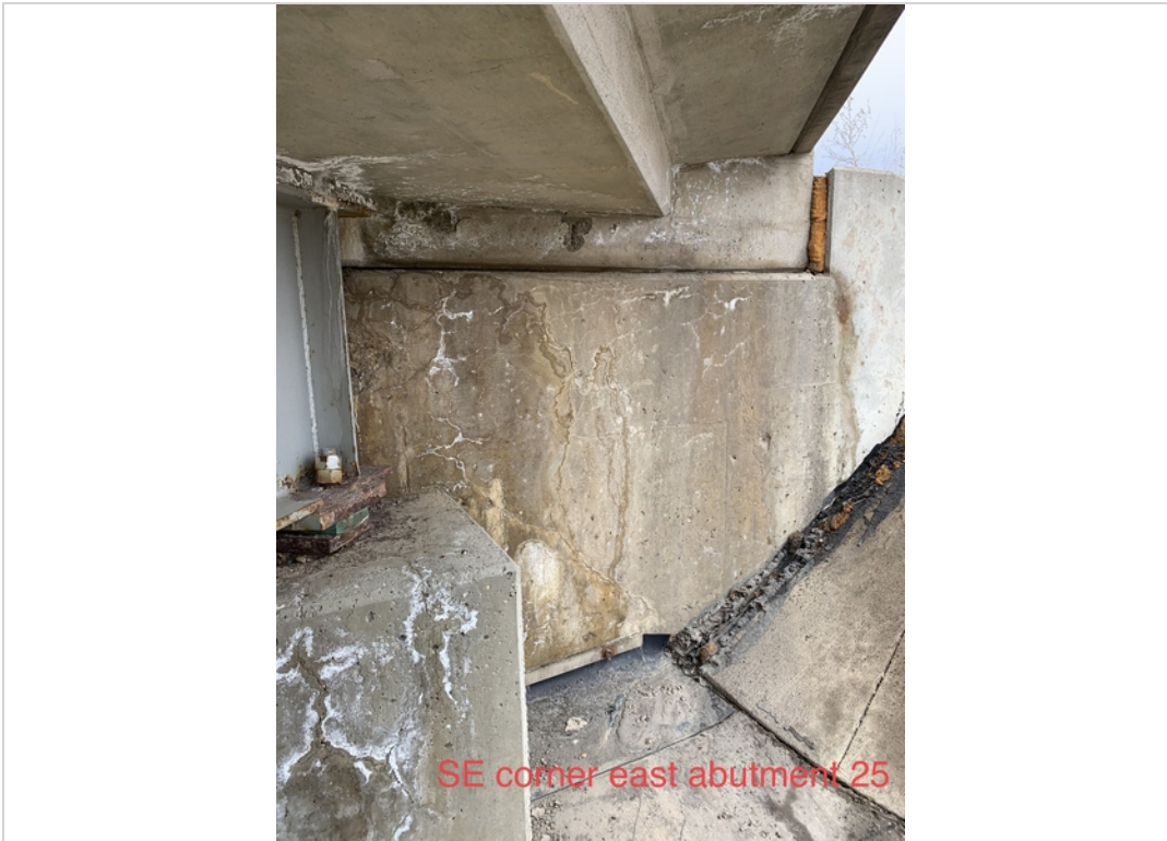
SE corner east abutment cracks efflorescence (25)
