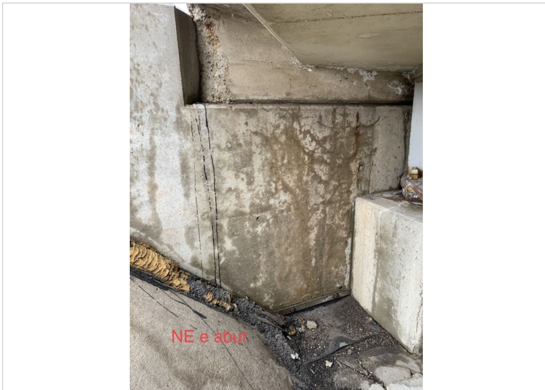
NE east corner east abutment cracks
