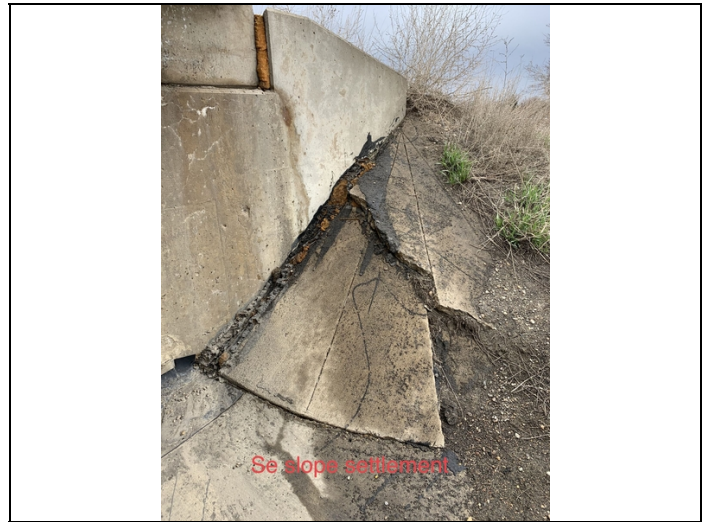
SE slope protection settlement
