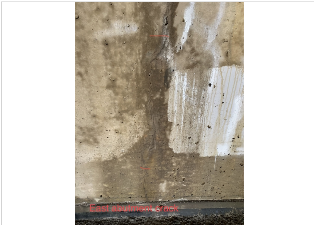
East abutment crack
