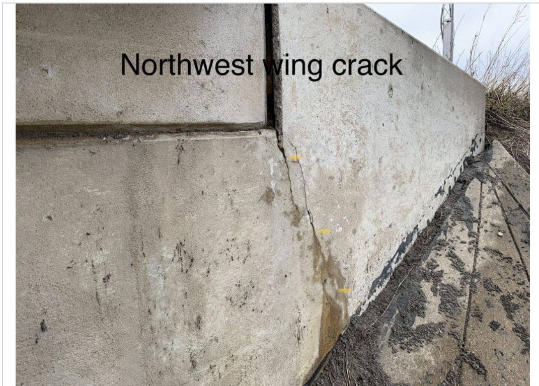
NW wing crack
