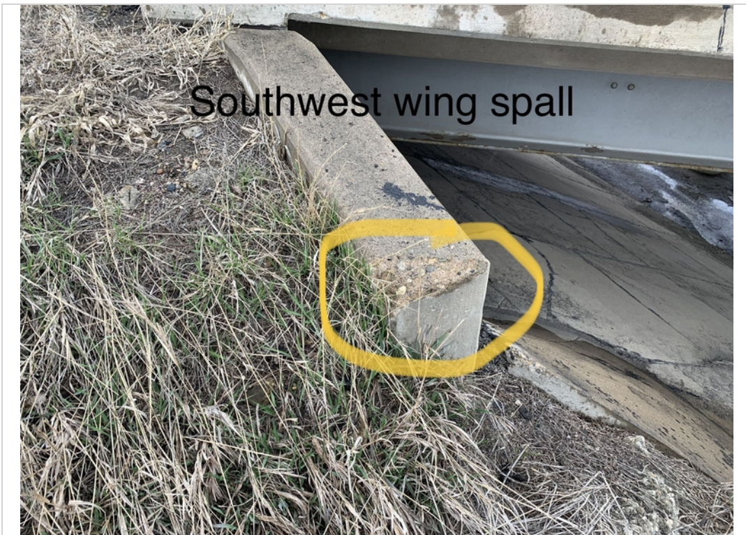
SW wing spall
