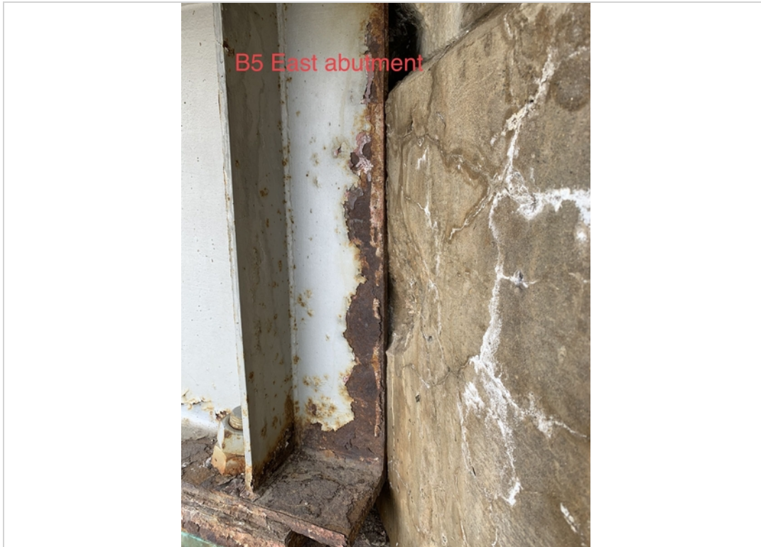
Beam 5 east abutment ,backwall spall, beam touching
