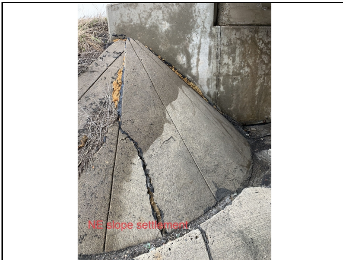
NE corner slope protection settlement
