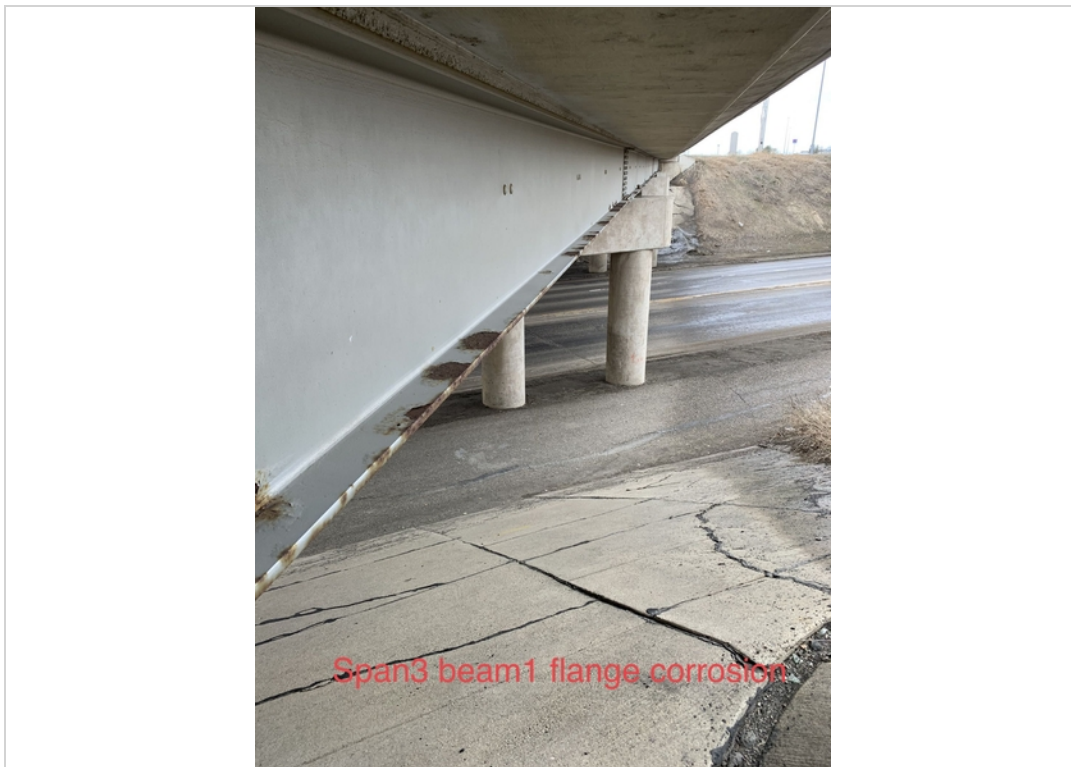
Span3 beam 1 bottom flange corrosion
