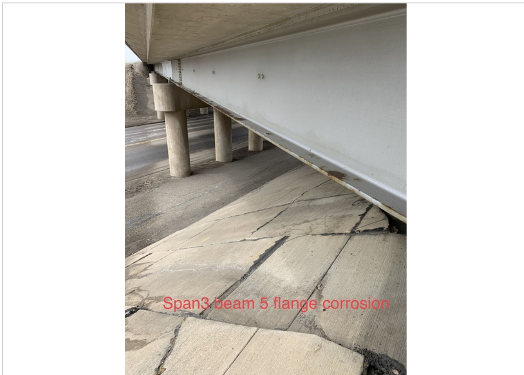
Span 3 beam 5 flange corrosion
