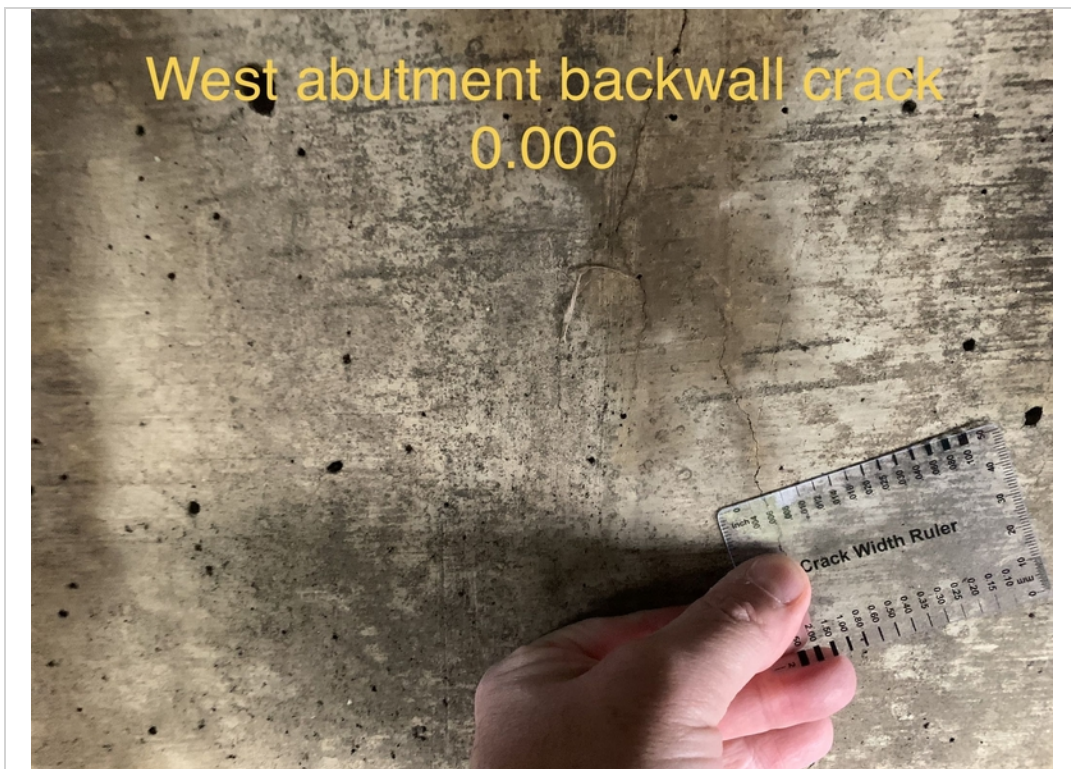
West abutment backwall crack .006
