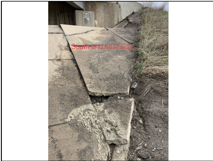
South end east slope protection broke and erosion
