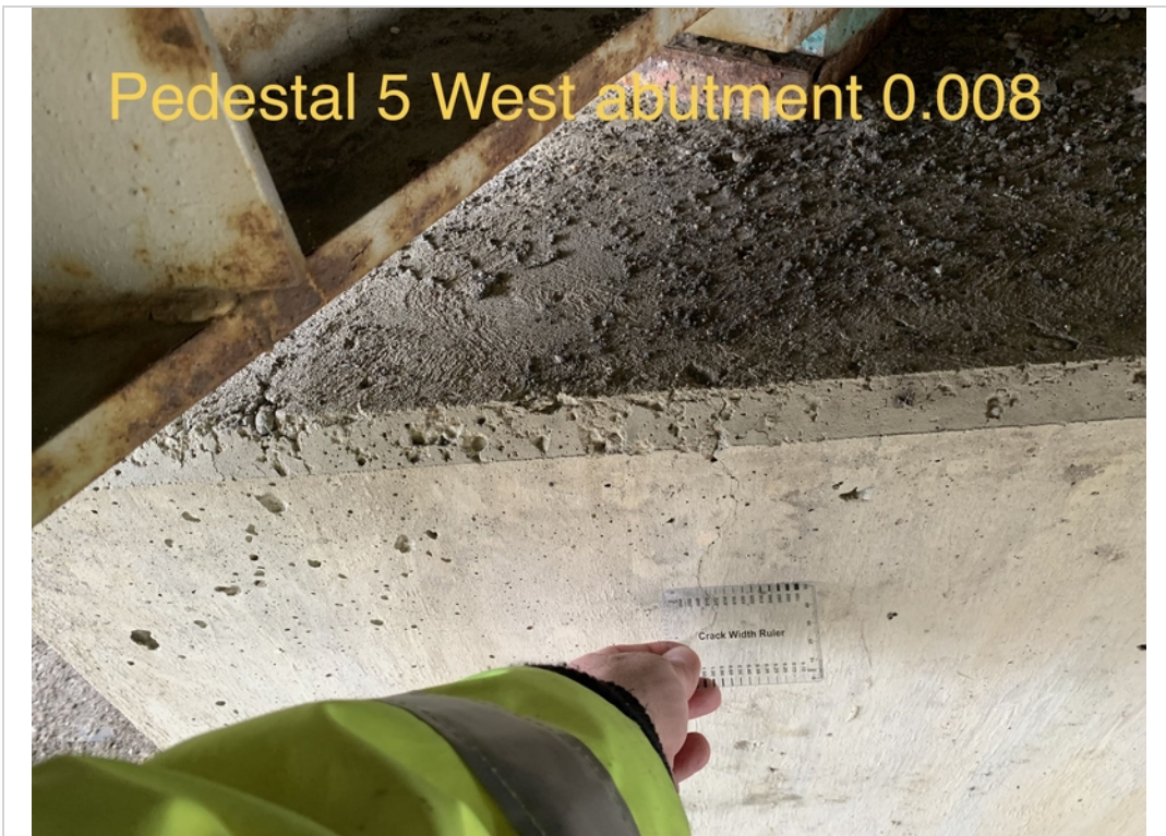
Ped 5 west abutment crack .008
