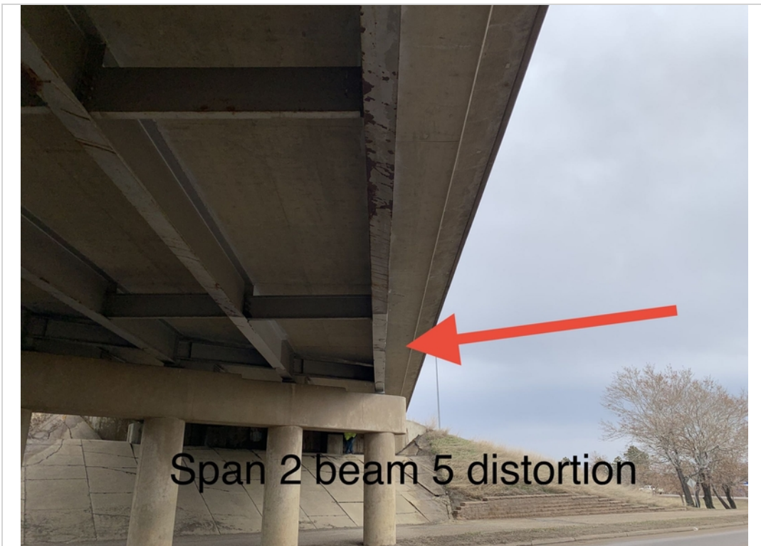
Span 2 beam5 distortion
