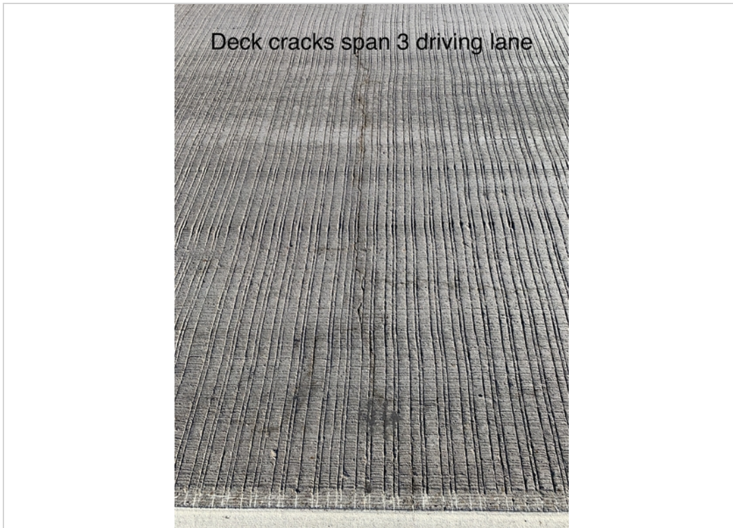
Deck cracks span 3 drive lane
