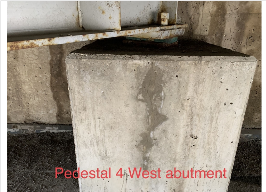
Ped 4 west abutment crack
