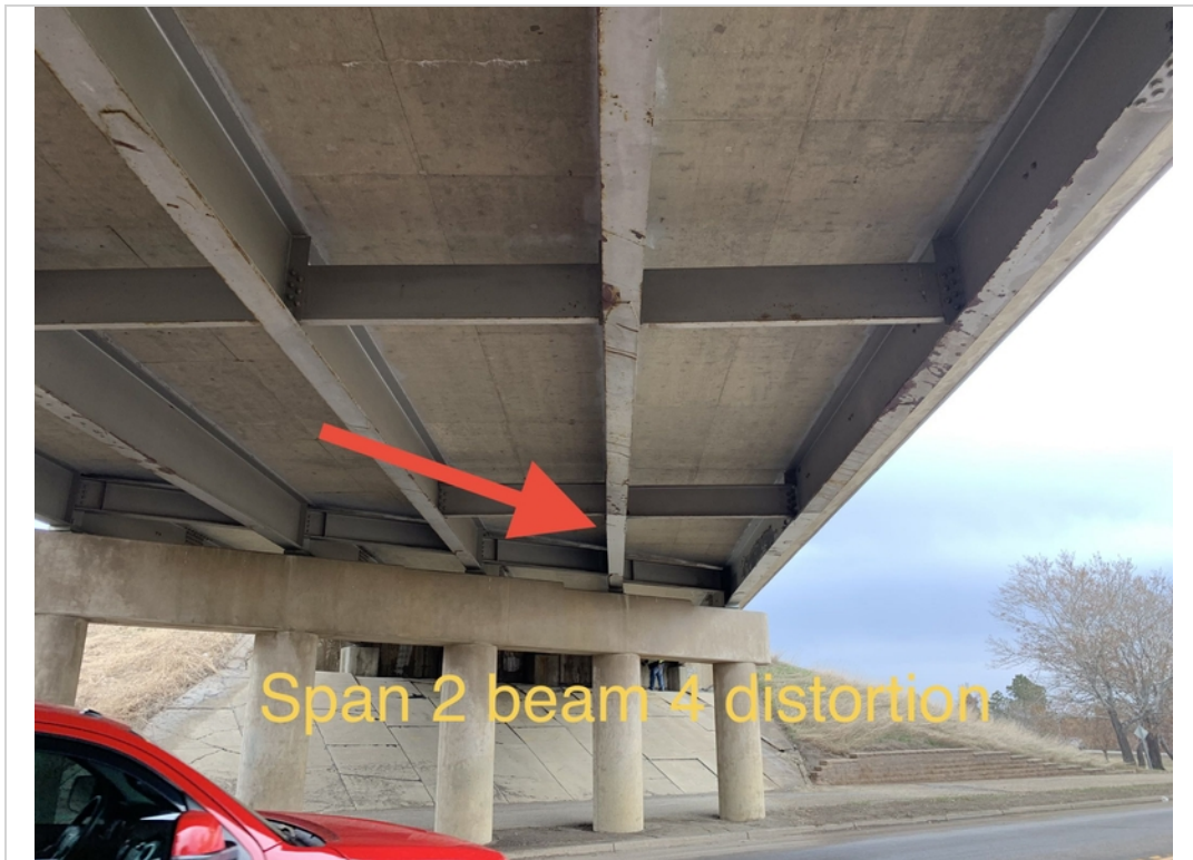
Span 2 beam 4 distortion
