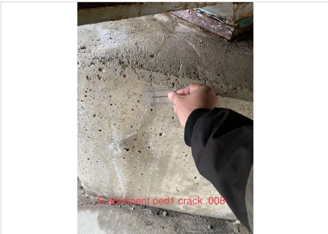
East abutment ped 1 crack .008
