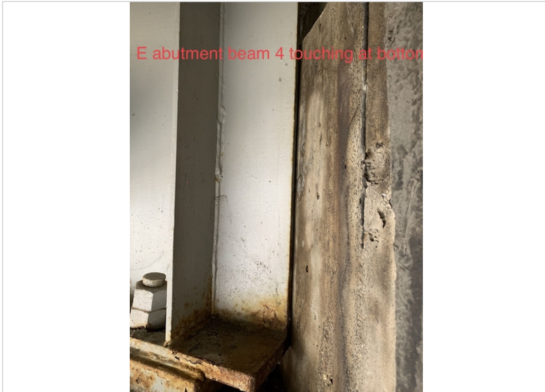
East abutment beam 4 touching abutment
