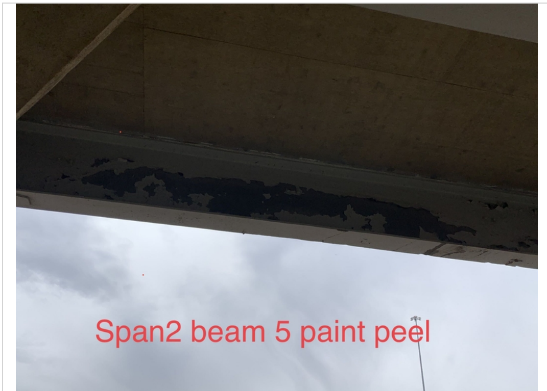
Span 2 beam 5 paint peel
