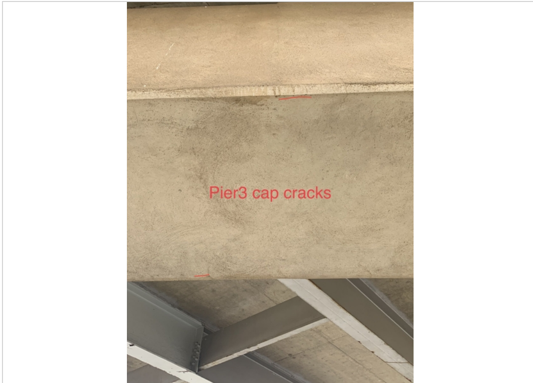
Pier 3 cap cracks
