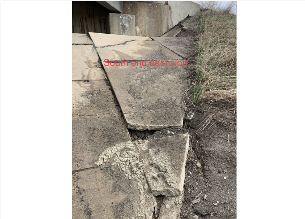
South end east slope protection broke and erosion
