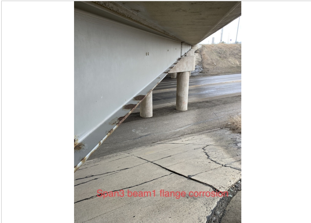
Span3 beam 1 bottom flange corrosion
