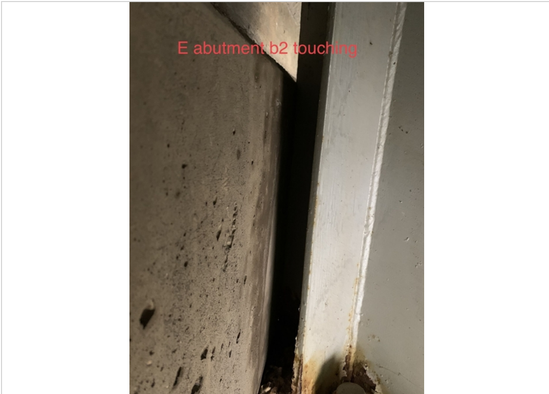
East abutment beam 2 touching abutment
