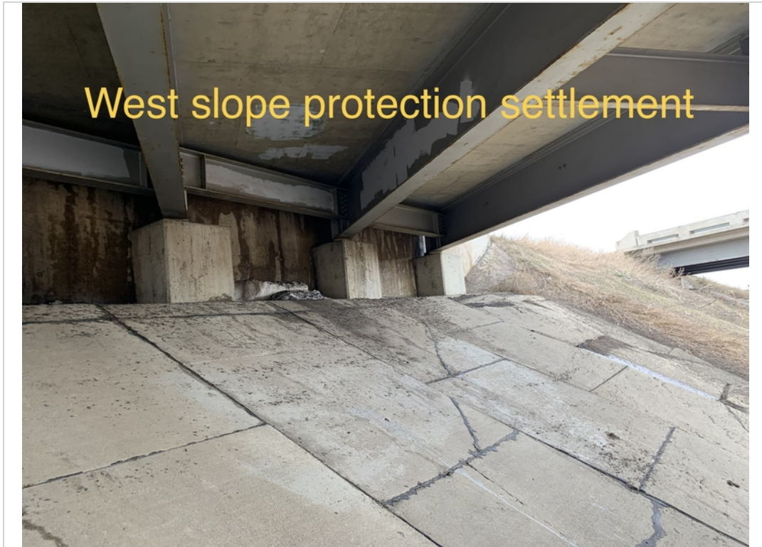
West slope protection settlement
