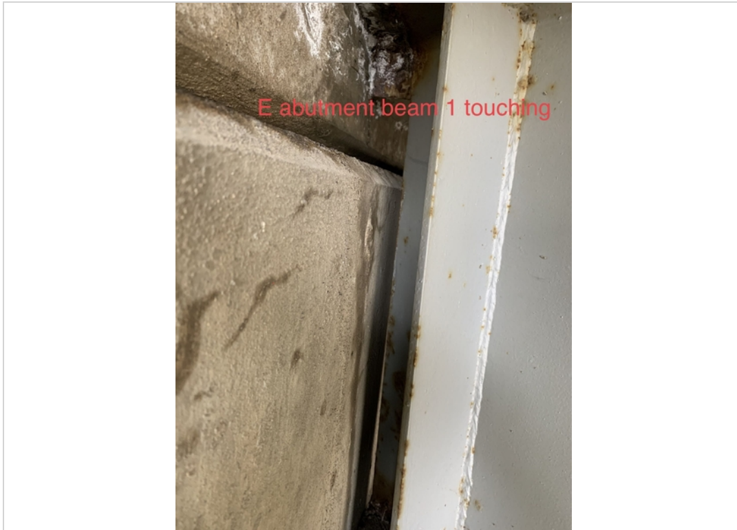
East abutment beam 1 touching abutment
