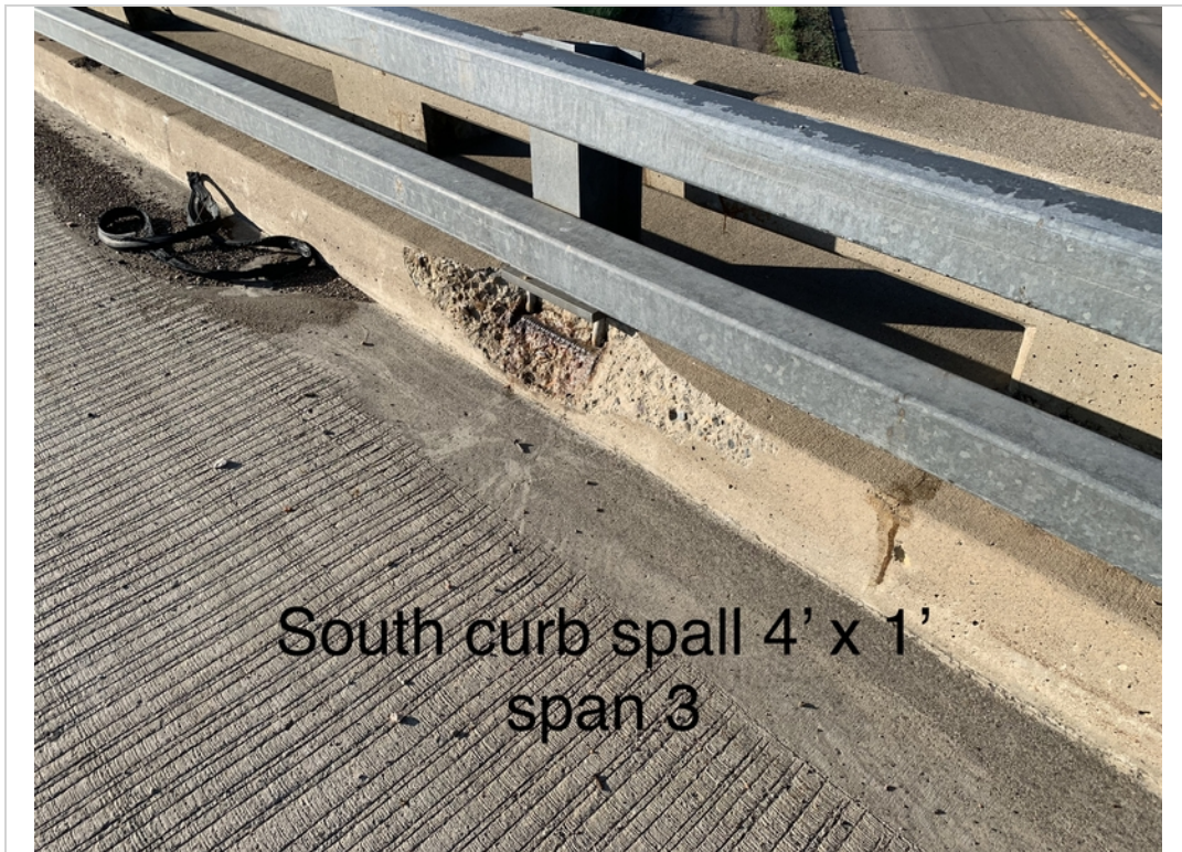
South curb spall 4'x1' span 3
