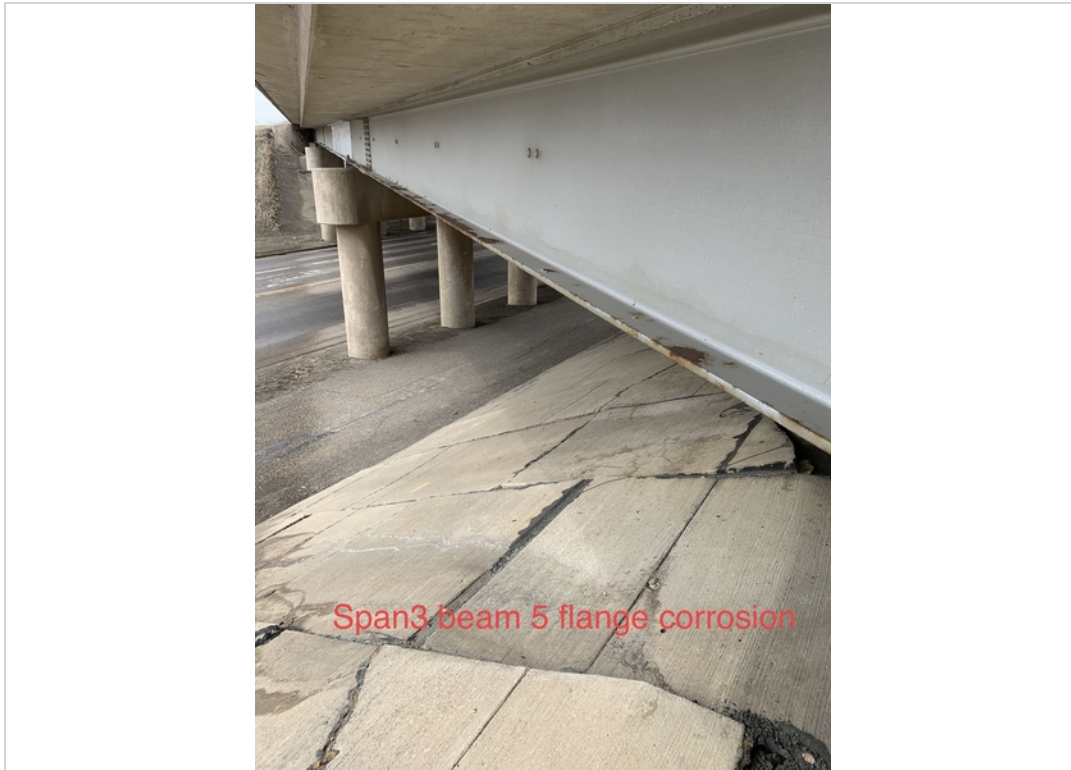
Span 3 beam 5 flange corrosion
