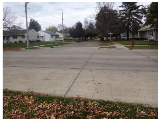
This intersection one block west of Ellis lacks curb ramps on the south side of 4th Avenue SE, painted crosswalks, and pedestrian signage.
