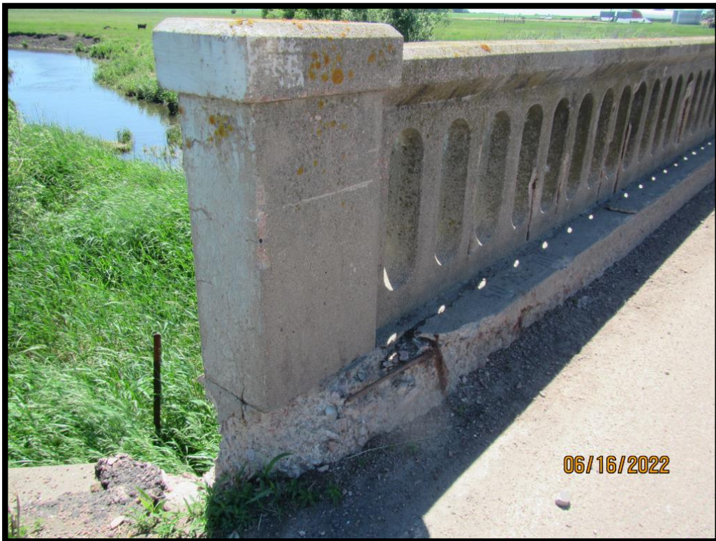
50-277-015_2022_10_CDI_SE Concrete Curb Spall with Exposed Rebar
