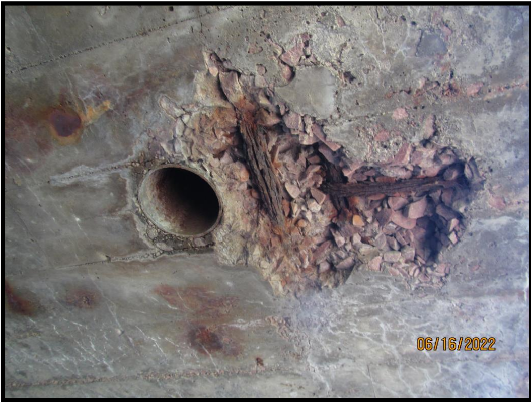
50-277-015_2022_20_CDI_Underside of Slab Span #4 Spall with Exposed Rebar at North Deck Drain
