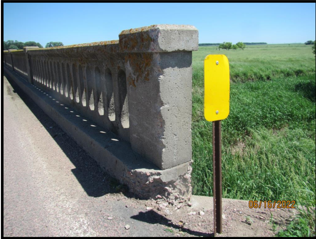
50-277-015_2022_9_CDI_SW Concrete Curb and Railing Spall
