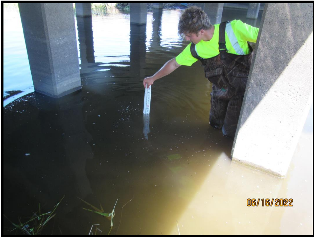
50-277-015_2022_27_CDI_Scour at West Bent between Column #1 and #2
