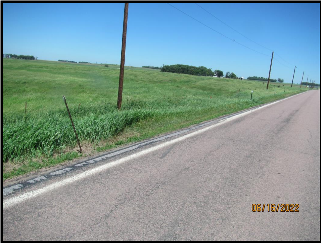
50-277-015_2022_5_CDI_1 st NE Approach Delineator Bent
