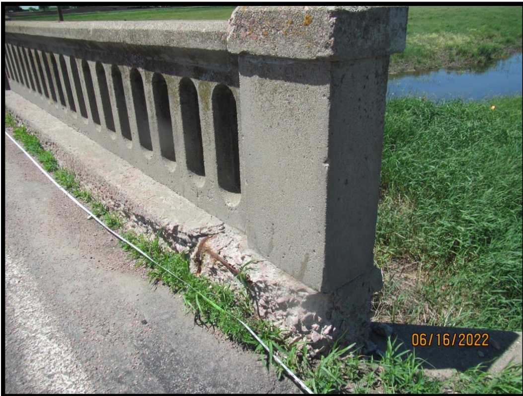
50-277-015_2022_12_CDI_NE Concrete Curb Spall with Exposed Rebar
