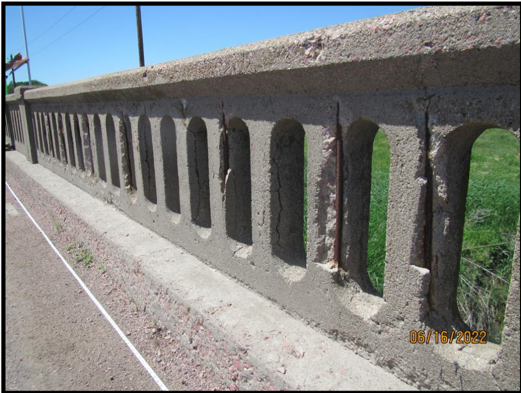
50-277-015_2022_16_CDI_Typical Concrete Railing Spalling with Exposed Rebar
