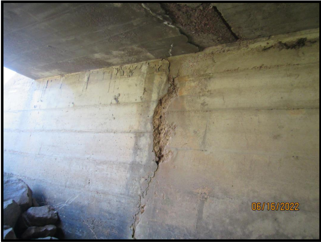
50-216-015_2022_21_CDI_NE Backwall Spall
