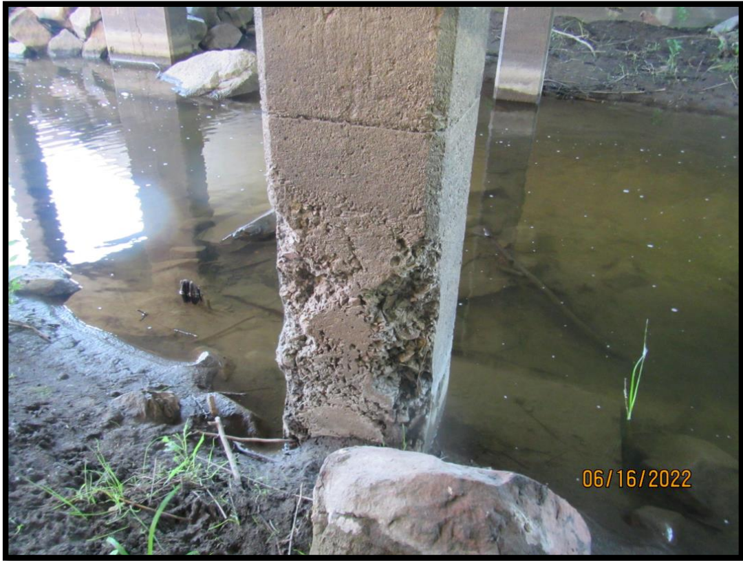
50-216-015_2022_23_CDI_West Bent Center Column Honeycombing
