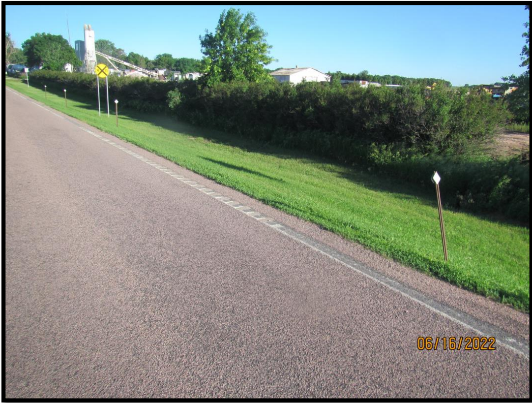
50-216-015_2022_7_CDI_1 st NW Approach Delineator Slightly Bent
