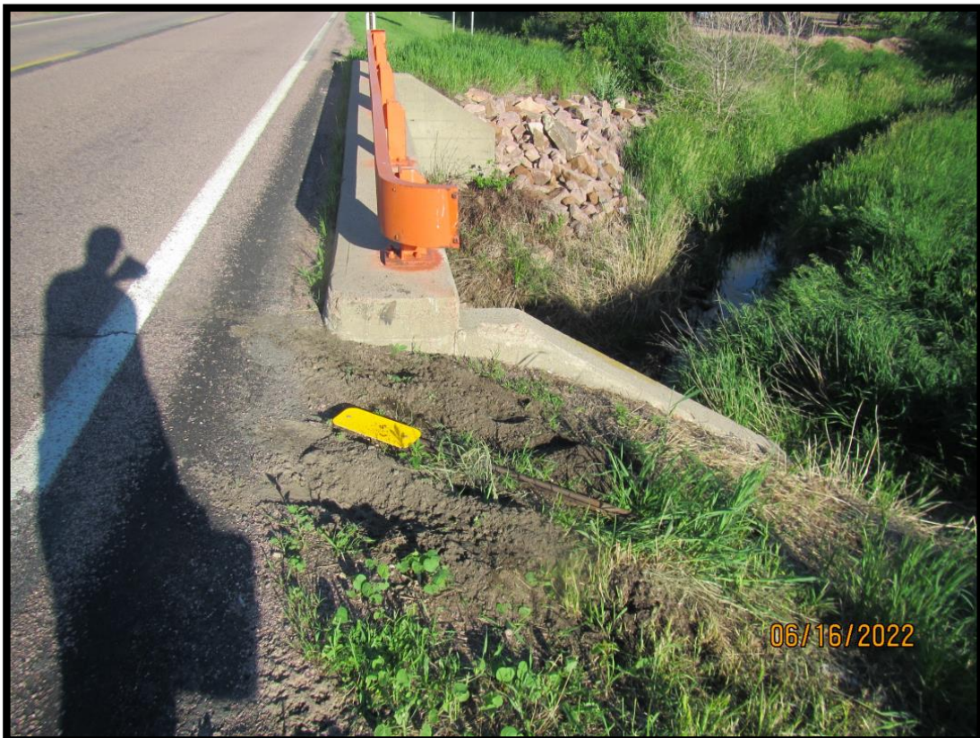
50-216-015_2022_6_CDI_NE Object Marker Damaged and on Ground
