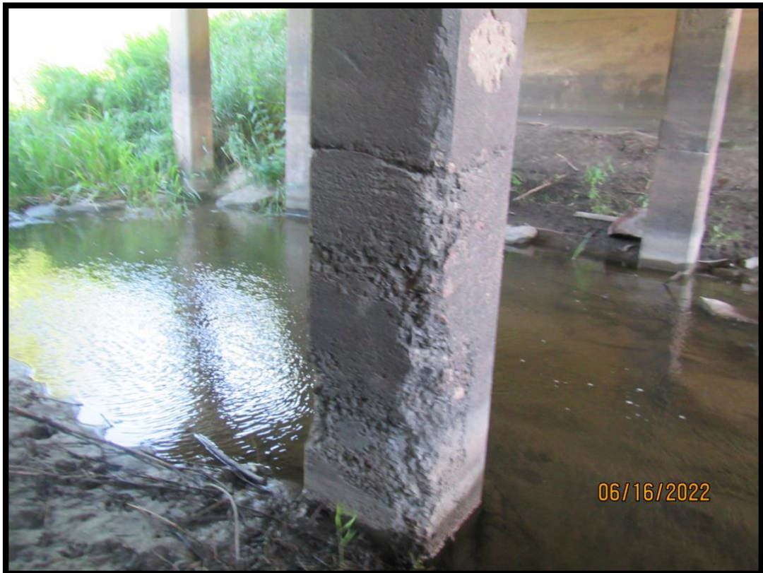
50-216-015_2022_24_CDI_East Bent Center Column Honeycombing
