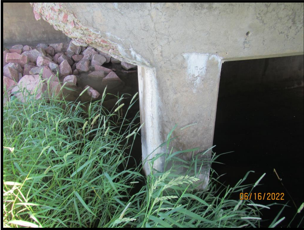
50-219-015_2022_25_CDI_Center Bent South Column Efflorescence Buildup
