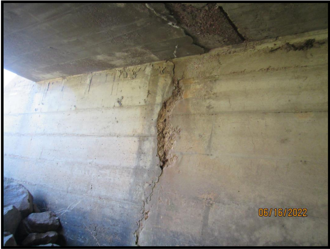
50-216-015_2022_21_CDI_NE Backwall Spall
