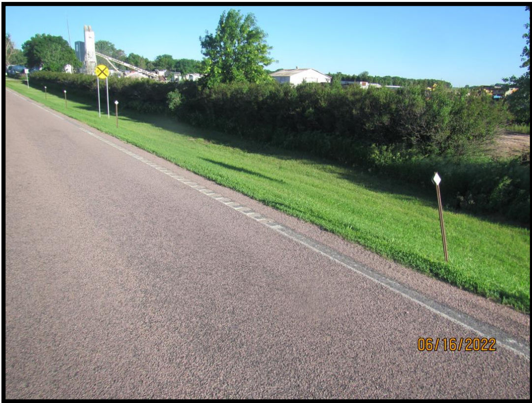
50-216-015_2022_7_CDI_1 st NW Approach Delineator Slightly Bent
