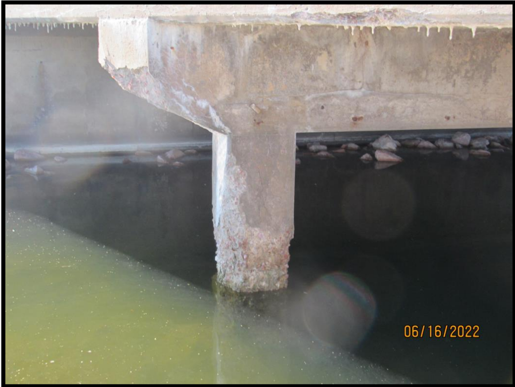
50-219-015_2022_24_CDI_North Bent Column Scaling
