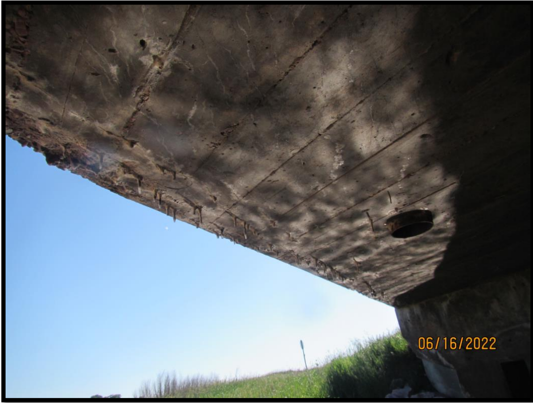
50-219-015_2022_19_CDI_Underside of North Edge of Slab in West Span with Stalactites
