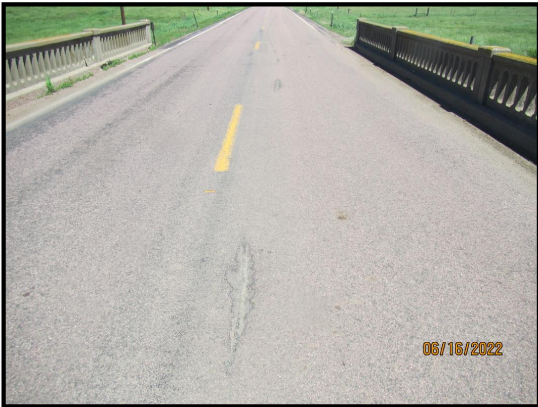
50-277-015_2022_8_CDI_Bituminous Overlay Gouges in Eastbound Lane
