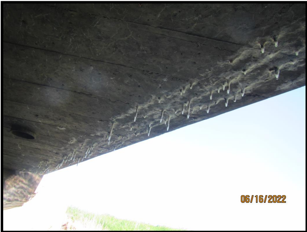
50-219-015_2022_20_CDI_Underside of North Edge of Slab in East Span with Stalactites
