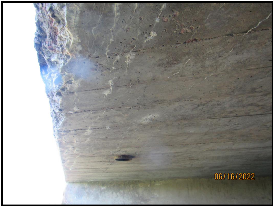
50-219-015_2022_18_CDI_Underside of South Edge of Slab in East Span with Stalactites
