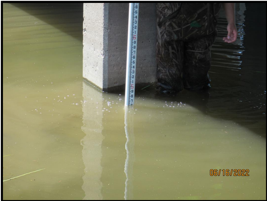
50-277-015_2022_28_CDI_Scour at Center Bent Column #1 (South)
