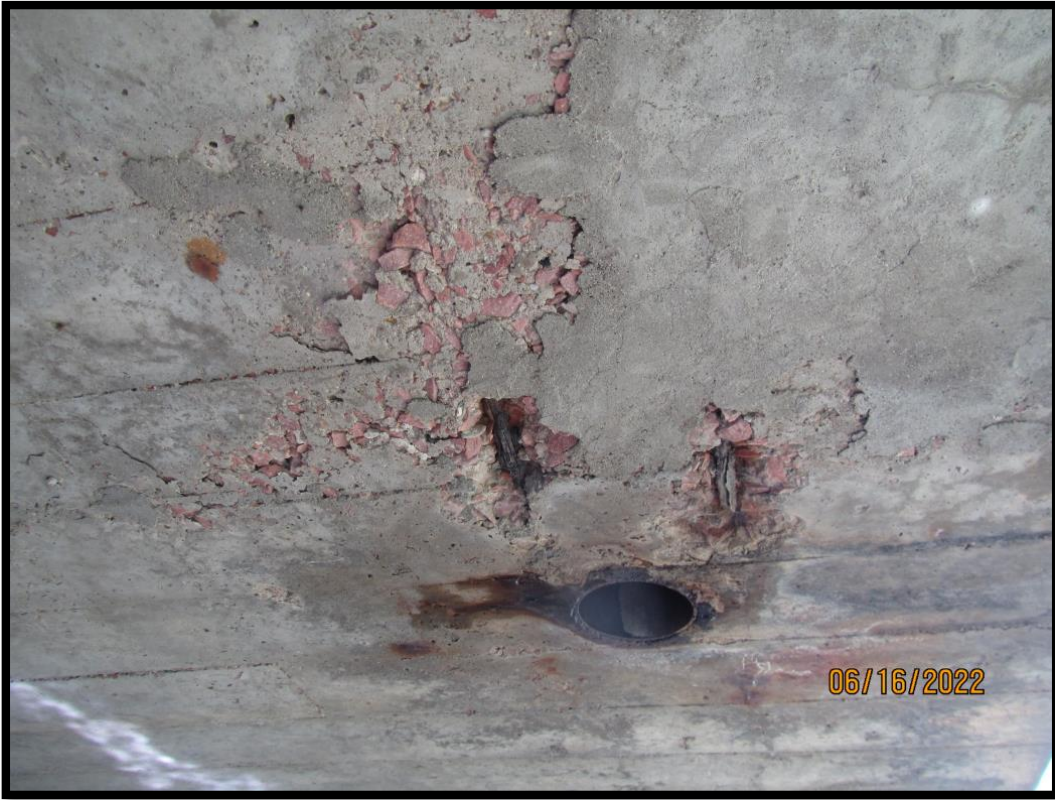
50-277-015_2022_19_CDI_Underside of Slab Span #4 Spall with Exposed Rebar at South Deck Drain
