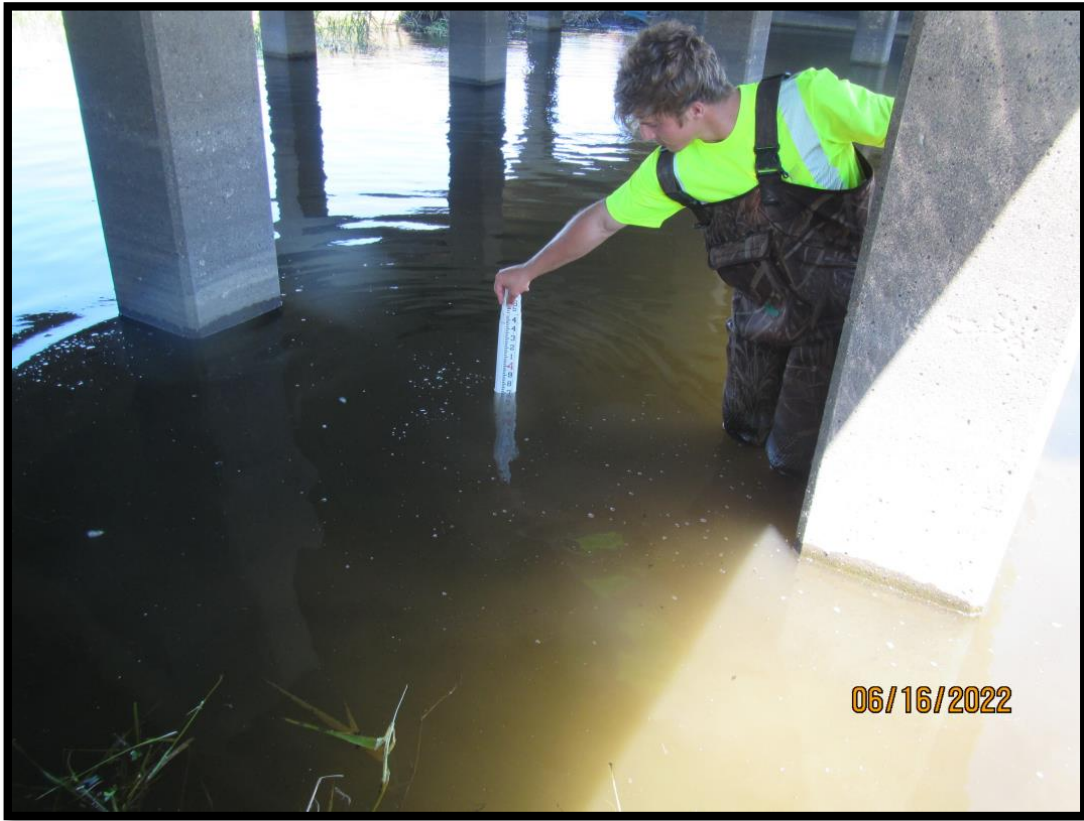
50-277-015_2022_27_CDI_Scour at West Bent between Column #1 and #2
