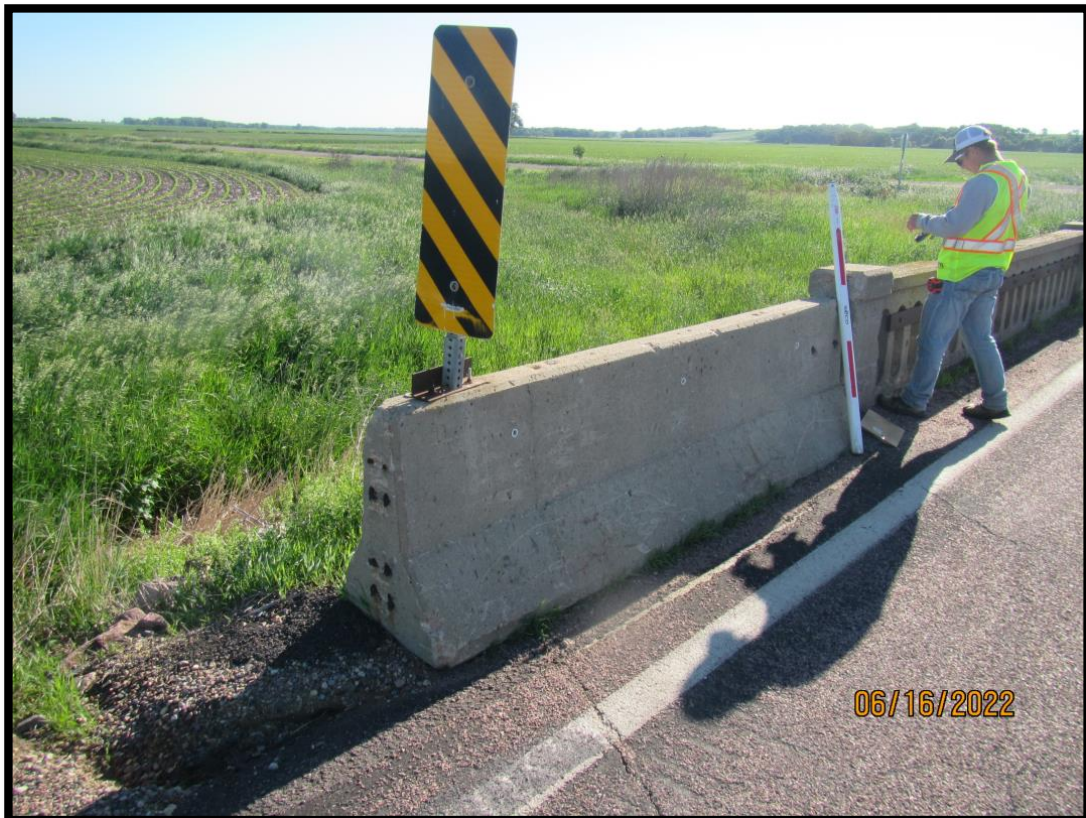
50-219-015_2022_14_CDI_NW Portable Concrete Jersey Barrier
