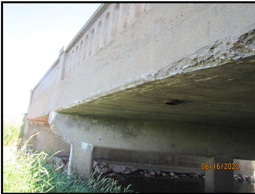
50-219-015_2022_21_CDI_South Edge of Slab with Efflorescence and Minor Stalactites
