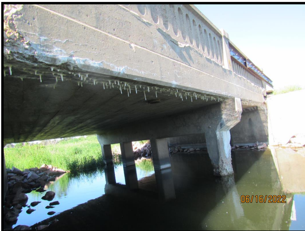
50-219-015_2022_22_CDI_North Edge of Slab with Active Stalactite Dripping
