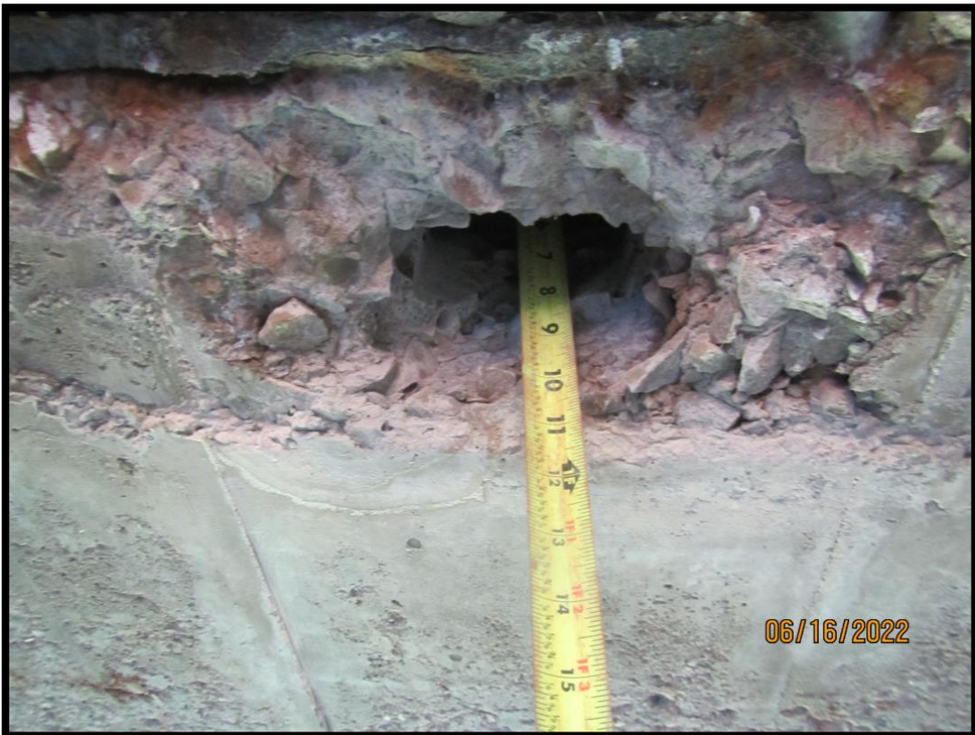
50-216-015_2022_18_CDI_Hole in underside of Slab, South side of West Span
