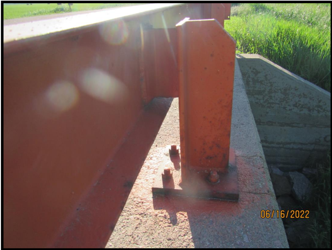
50-216-015_2022_11_CDI_Typical Rail Post Condition
