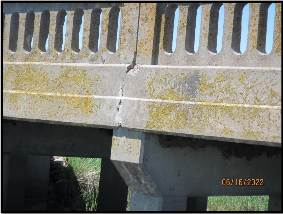
50-277-015_2022_13_CDI_South Curb and Slab Vertical Crack over Center Bent
