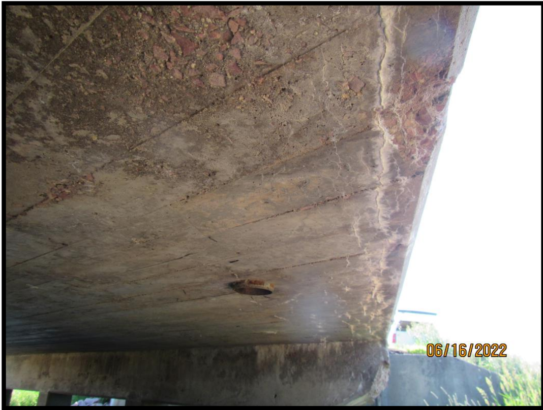
50-219-015_2022_17_CDI_Underside of South Edge of Slab in West Span with Stalactites
