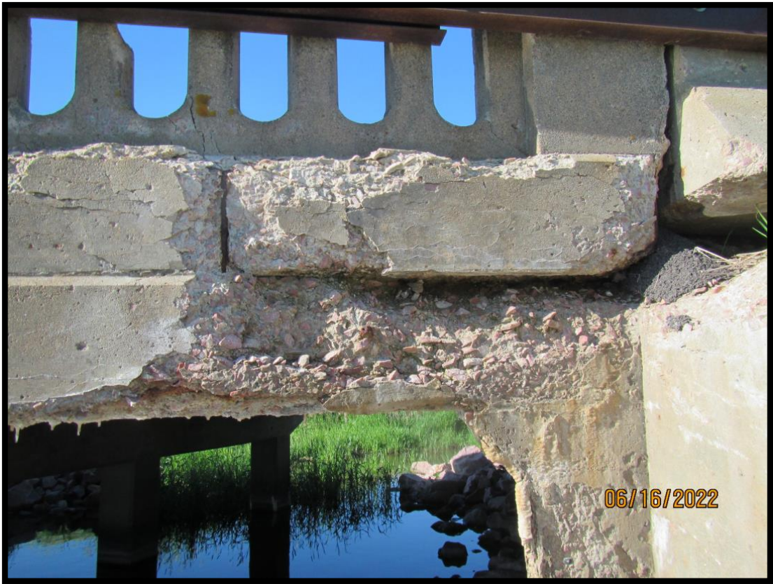
50-219-015_2022_9_CDI_NW Slab and Curb Edge Deterioration and Damage
