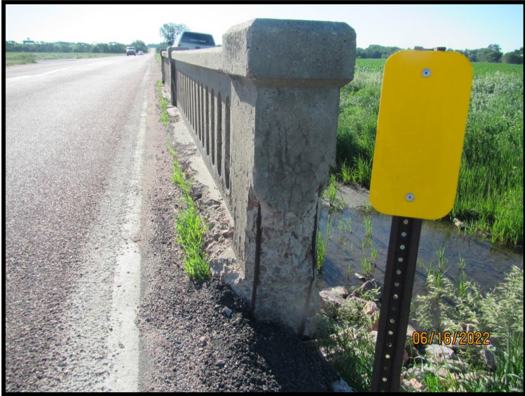
50-219-015_2022_15_CDI_SW Rail end Spall with Exposed Rebar
