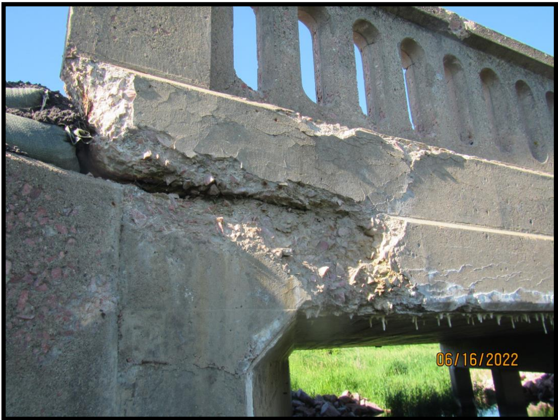
50-219-015_2022_10_CDI_NE Slab and Curb Edge Deterioration
