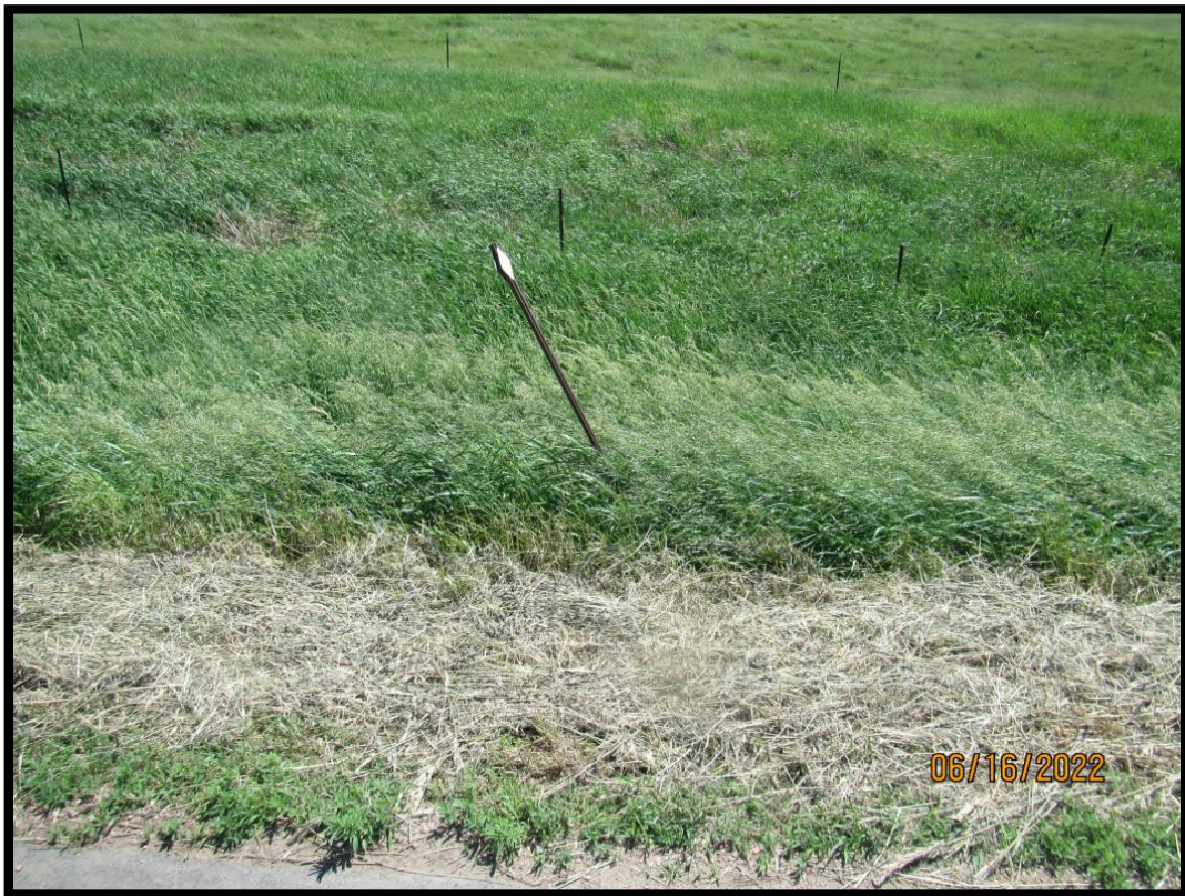
50-277-015_2022_6_CDI_4 th SW Approach Delineator Bent
