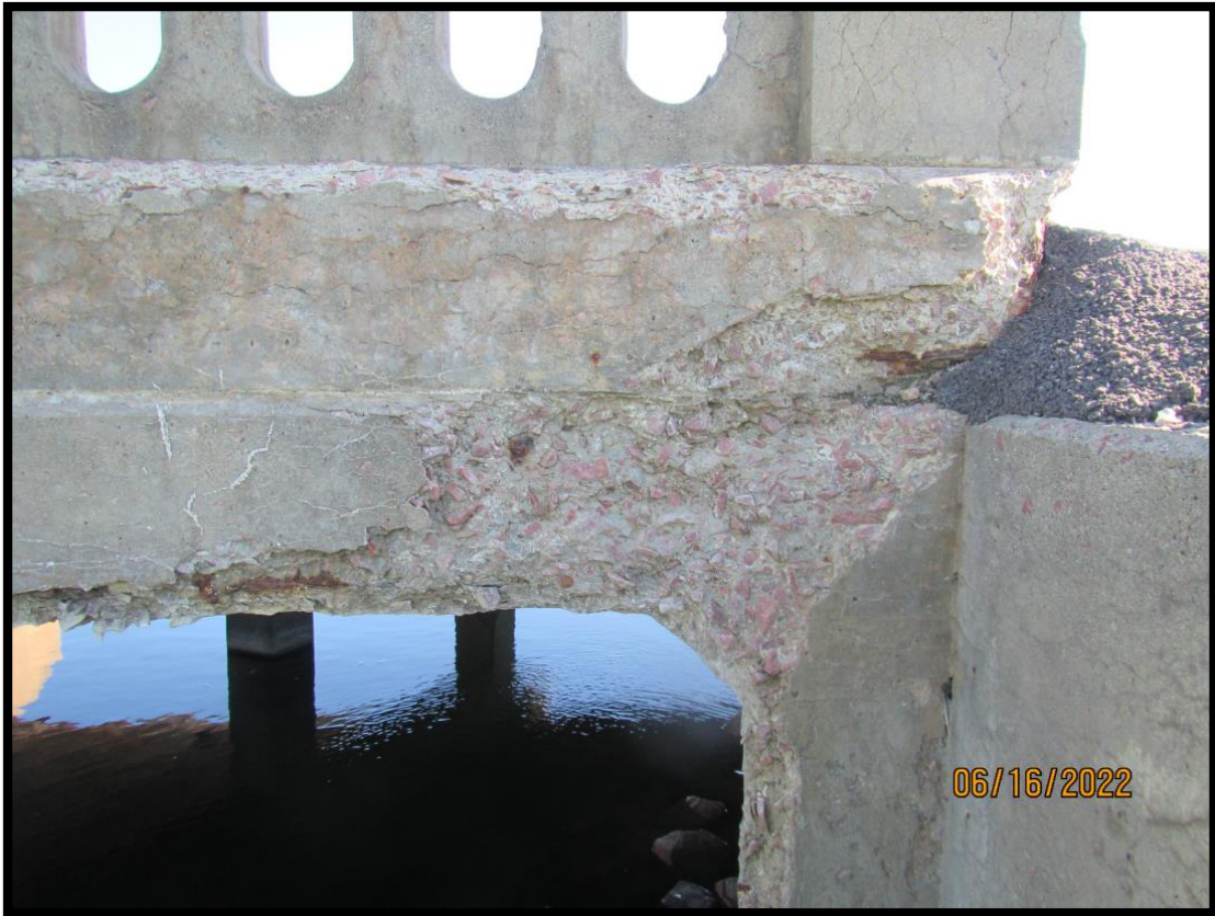
50-219-015_2022_11_CDI_SE Slab and Curb Edge Deterioration
