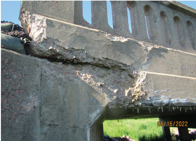
Figure 5 50-277-015 Deck & Curb Vertical Crack over Center Pier
