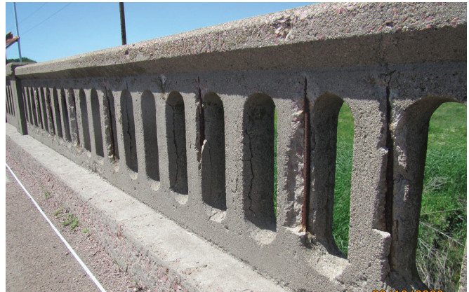
Figure 11 50-277-015 Concrete Railing Spall and Exposed rebar
