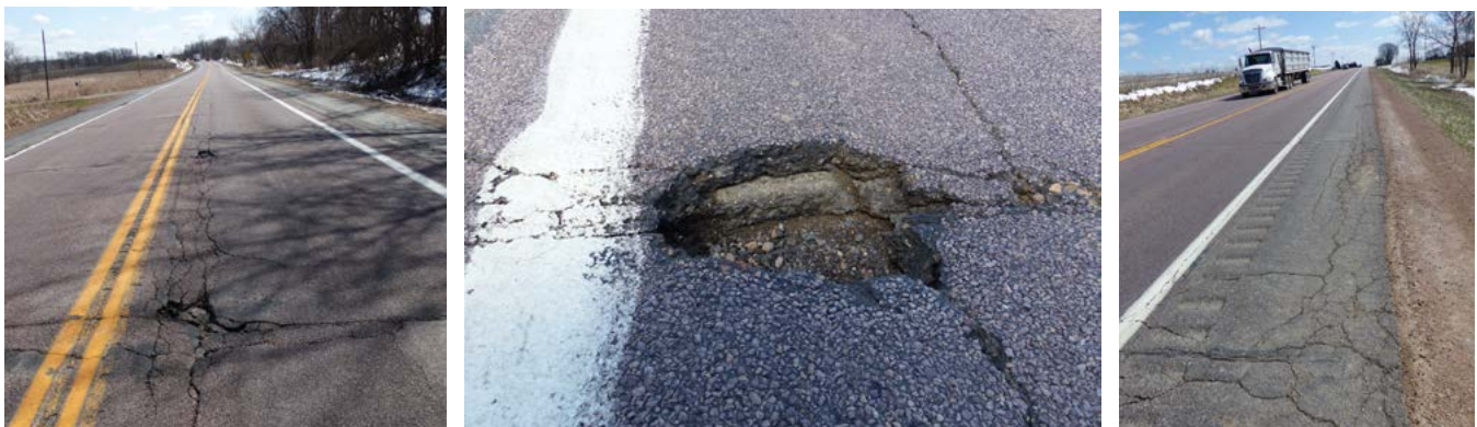
Figure 13 Examples of poor pavement conditions on the corridor
