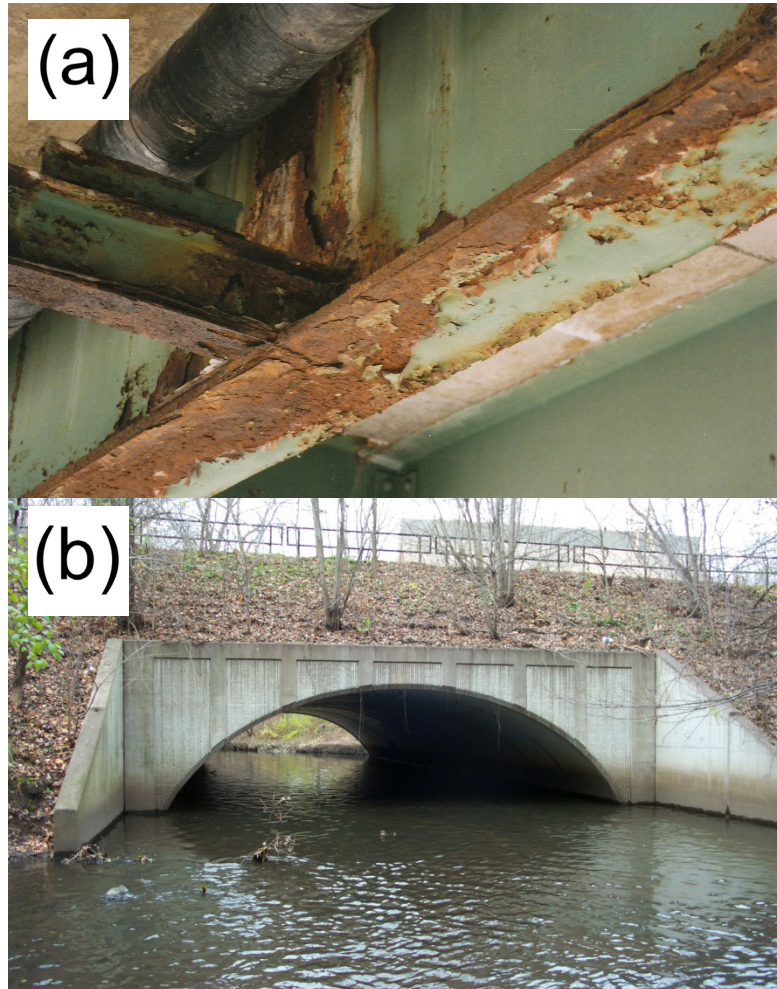
Figure 6-6: (a) Corrosion on a Bridge Structure Element (b) Large Culvert
